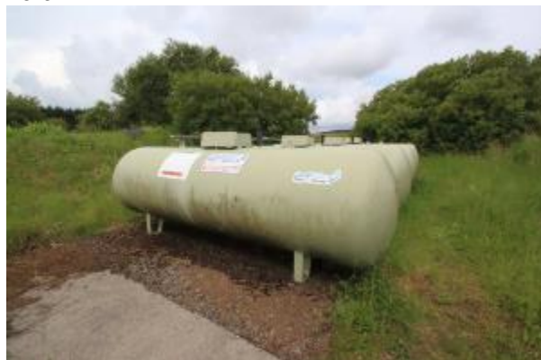
Photo 28: gas tanks over hardstanding, looking north
