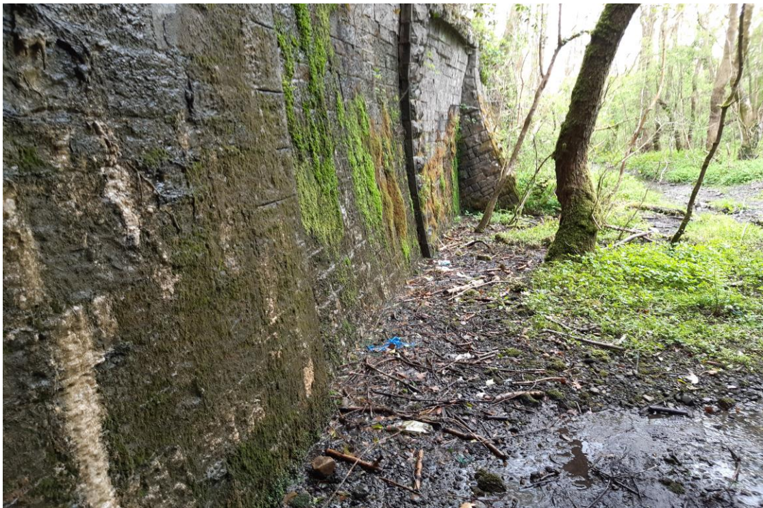
Plate 8 Photos viewing groundwater seepage through the masonry of the bridge which crosses over the former Aberdare to Merthyr railway line - 7.
