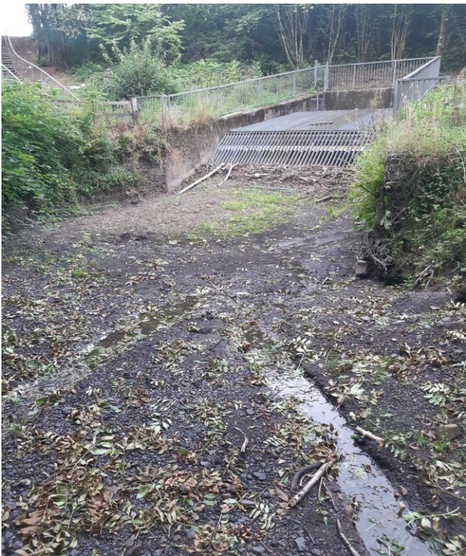
Plate 24 Photo showing heavily silted Nant Cannaid and the culvert beneath the A470 - 17
