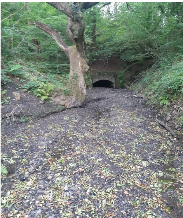
Plate 23 Photo showing heavily silted Nant Cannaid and the culvert beneath the A470 - 17
