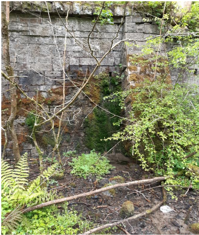
Plate 9 Photos viewing groundwater seepage through the masonry of the bridge which crosses over the former Aberdare to Merthyr railway line - 7.
