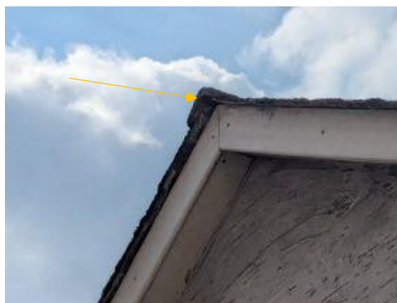
PRF – Gap under ridge tile (onto uPVC surface)
