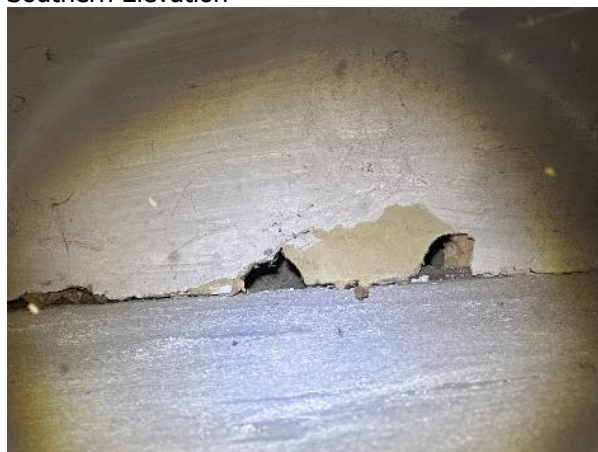
Photo 20: Gaps on the Ceiling of the Porch on the Southern Elevation
