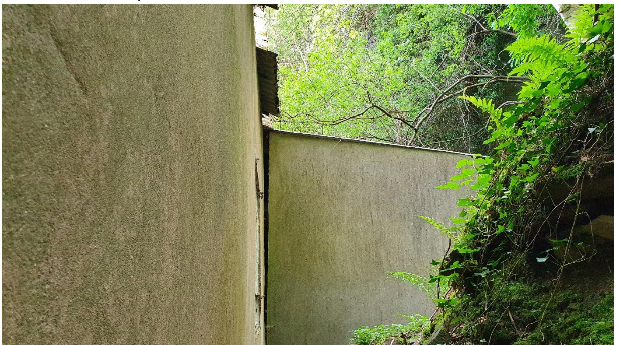
Photo 7: There is a small lean-to storage room along the western aspect. The mortar along the joint is severely damaged and part of the building has pulled away from the wall. Light is clearly visible on the other side of the crack. The crack offers limited roosting potential for crevice dwelling bats. The space between the two walls was simple to inspect, it was heavily cobwebbed and no bats or evidence of bats was found.
