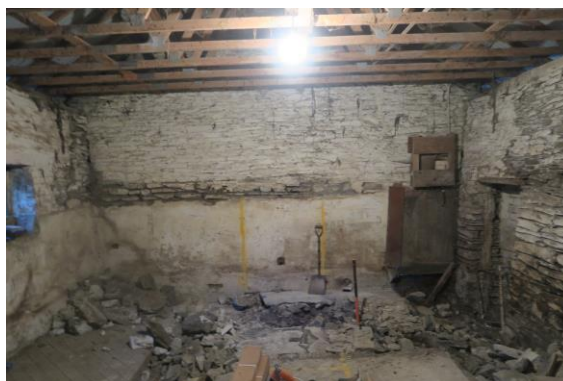
SOUTH ELEVATION INTERNAL: NOTE BOARDED OVER OPENING AND WITH STRAIGHT JOINTS AT CORNERS– OPENING TO BE MADE NARROWER AND NEW WINDOW
