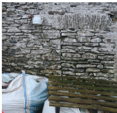
EAST ELEVATION / SOUTH END: NOTE INFILLED OPENINGS WITH STRAIGHT JOINT – SIDES OF OPENING TO BE BONDED TO INFILL:
