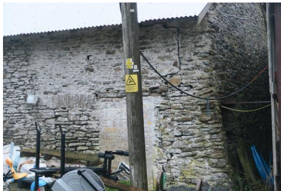
EAST ELEVATION / SOUTH END: NOTE INFILLED OPENINGS AND CRACK IN UPPER SECTION – SIDES OF OPENING TO BE BONDED TO INFILL AND CRACK TO BE REPAIRED BY INTRODUCING STONES BETWEEN WALL EACH SIDE:
