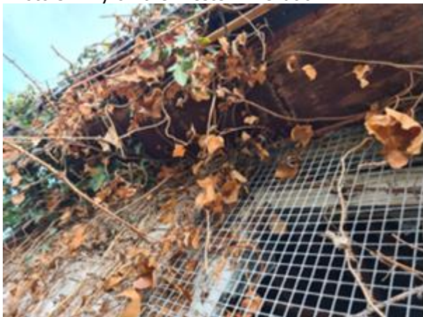
Photo 5: Ivy on the Western Elevation
