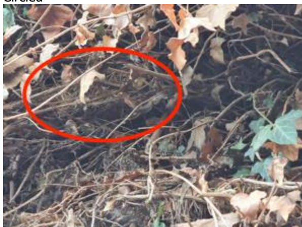
Photo 22: Defunct Nest, Northern Elevation, Circled
