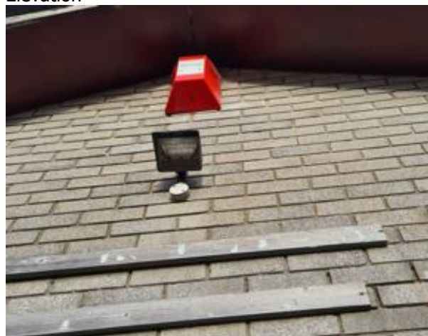
Photo 20: Smashed Security Light, on Southern Elevation
