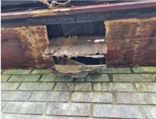
Photo 11: Broken Timber Soffit Box
