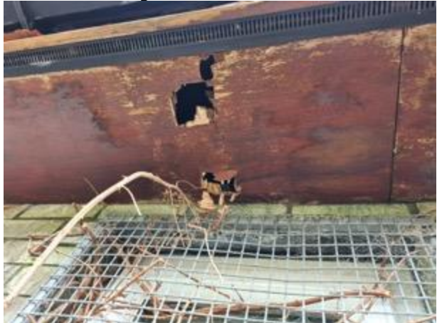
Photo 12: Damaged Timber Soffit Box
