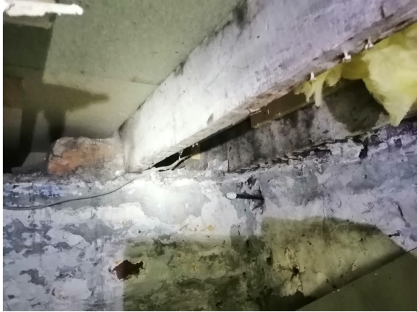
Storage room interior with crevices
