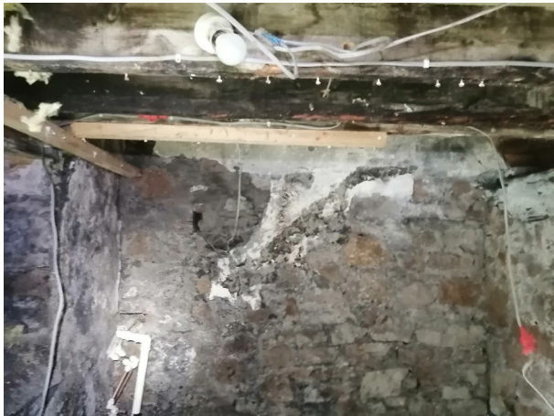
Storage room interior with crevices
