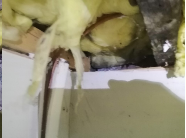
Storage room interior with crevices
