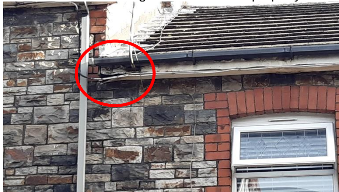
Damaged fascia and soffit covering on the NE corner of the gable end of property 32.
