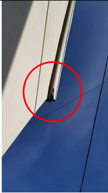
Fascia and soffit damaged on the front of property 30
