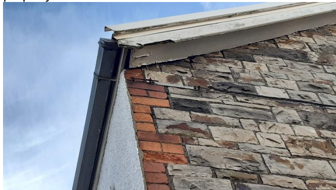
Damaged fascia and soffit covering on the NW corner of the gable end of property 32.
