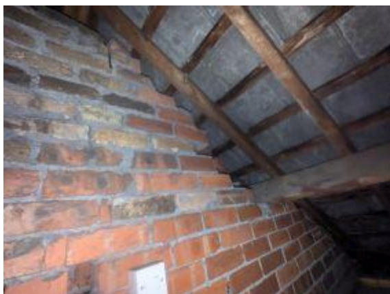
PRFs – Cavity above bitumen membrane.
