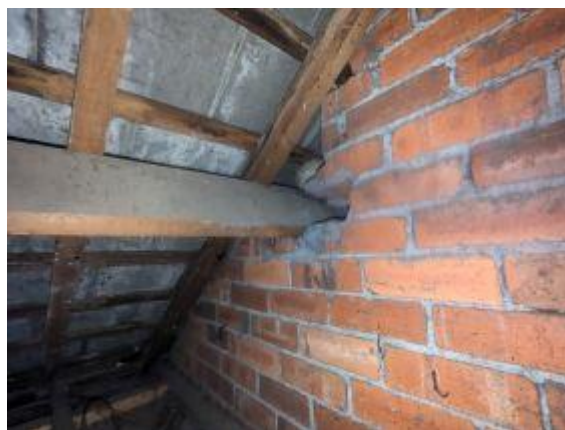
PRFs – Cavity above bitumen membrane.
