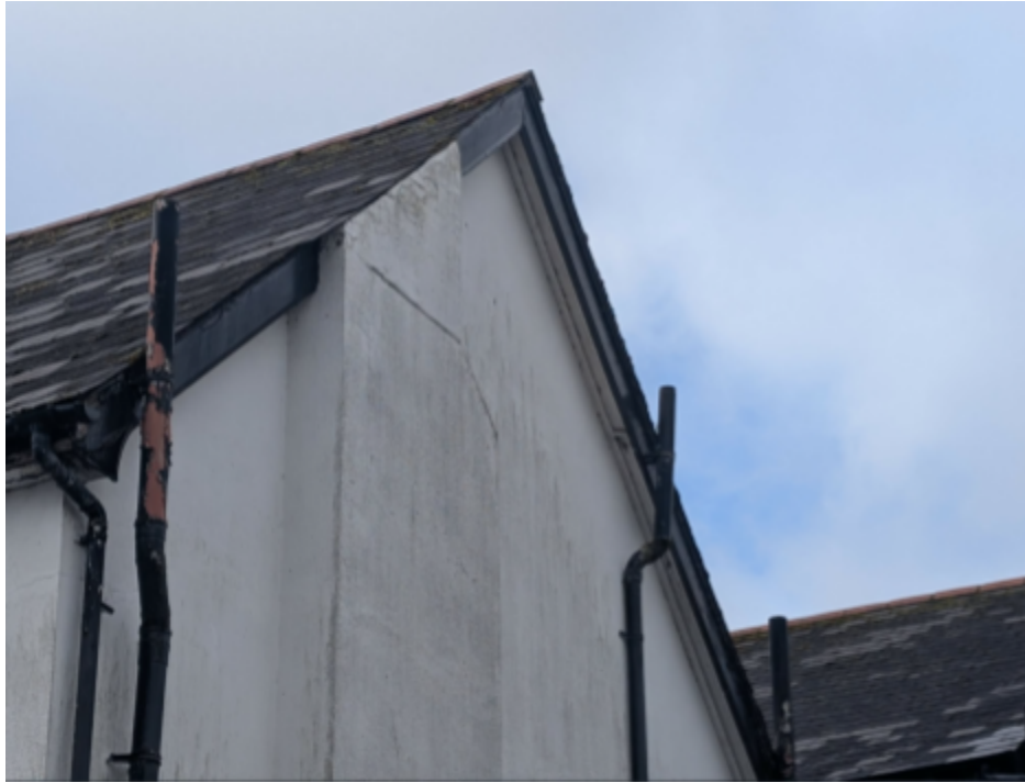
Plate 5- photograph of tight fitting soffits
