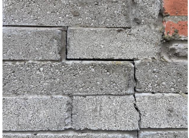
Photo 21: Large Crack in Breezeblock Section on Northern Elevation
