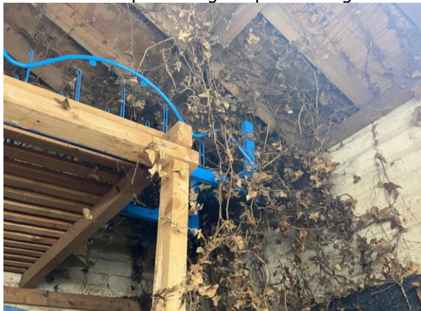
Photo 26: Example of Large Gaps With Vegetation
