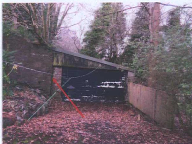
Figure 12: Garage (missing mortar in brickwork)
