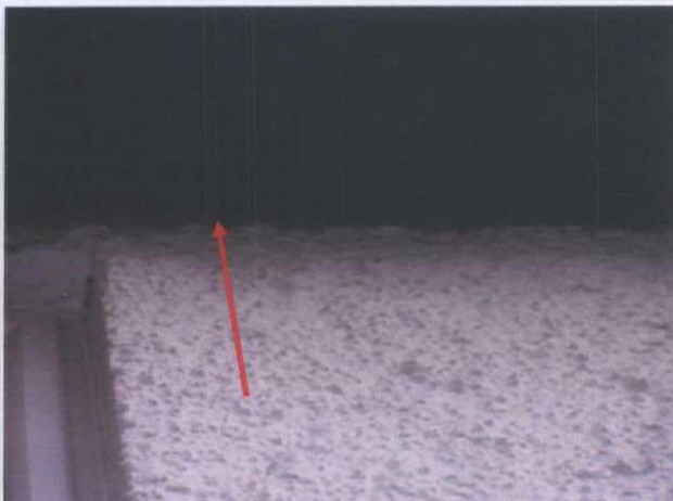
Figure 11: Gap between soffit box and wall
