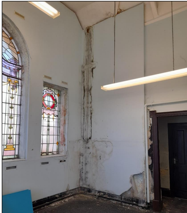
Plate 20. North-west corner of children's library, showing water damage.
