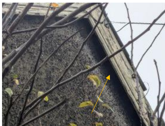
Northern elevation – PRF – Gap behind bargeboard.
