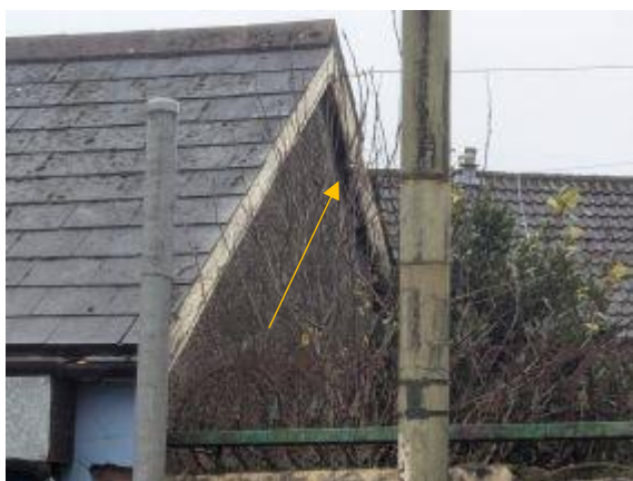
Northern elevation – PRF – Gap behind bargeboard.
