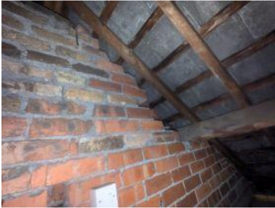
PRFs – Cavity above bitumen membrane.
