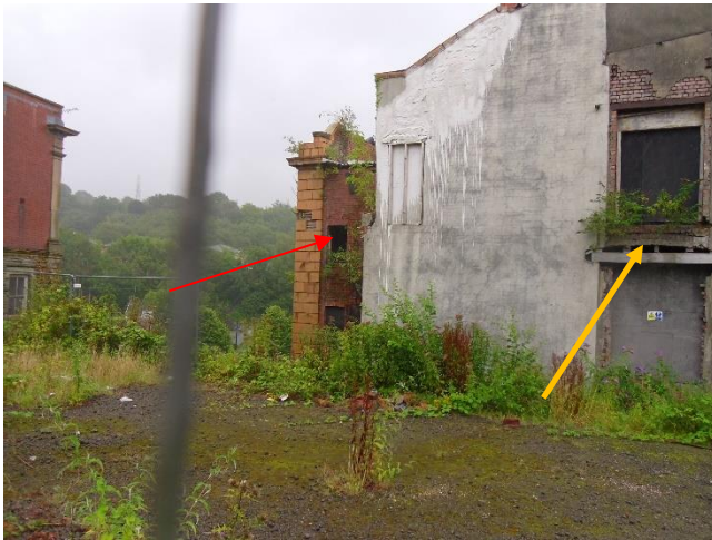
Figure 4 - Un-boarded window that lesser horseshoe bat accessed the building at the rear of the property (red arrow), suitable bat access feature (orange arrow)
