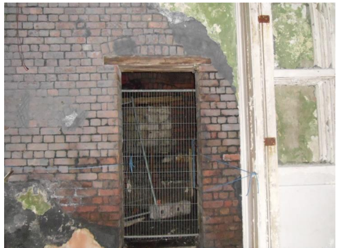
Figure 15 - Fenced off door at rear of building
