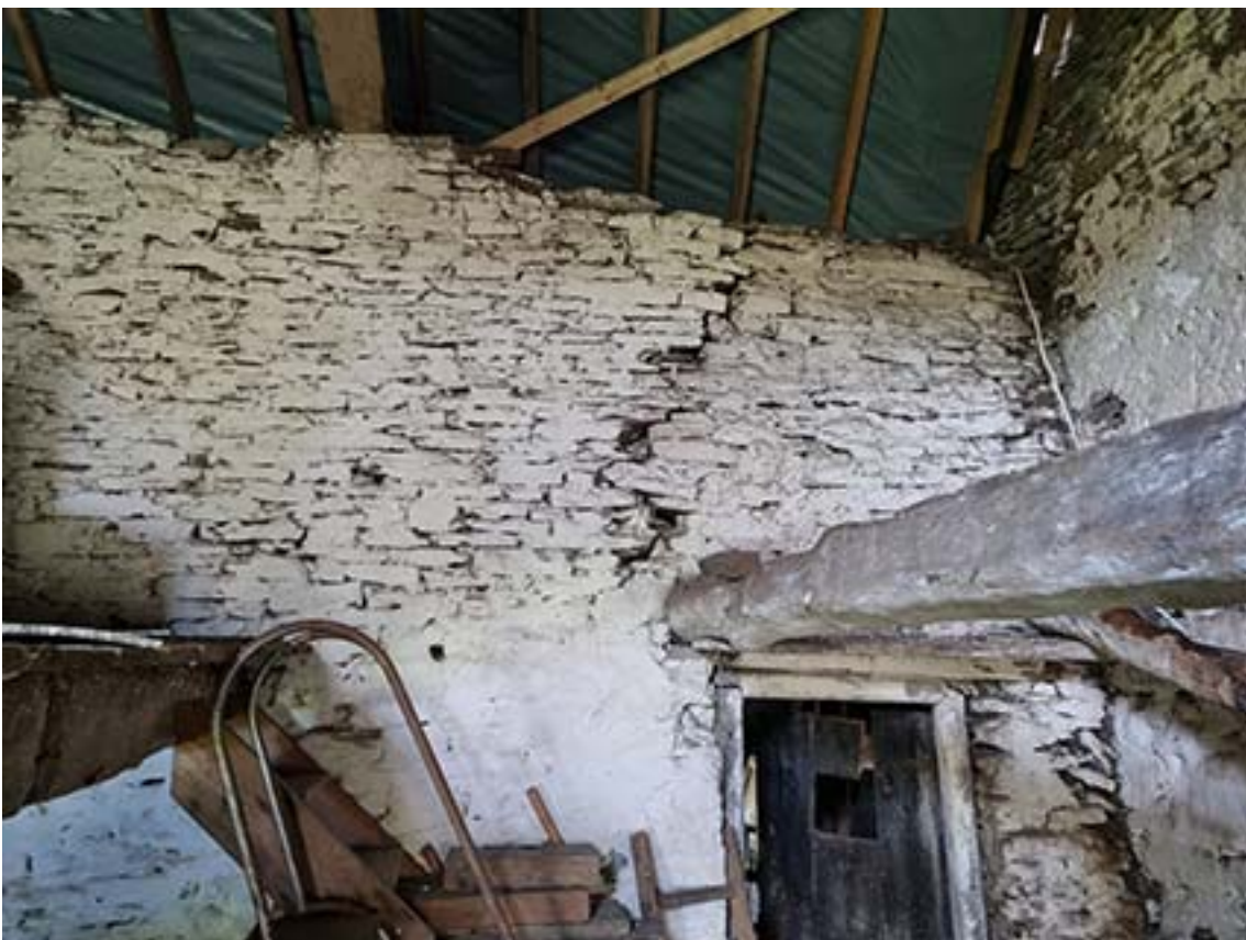
Photo of crack in internal wall and uneven wall plate level
