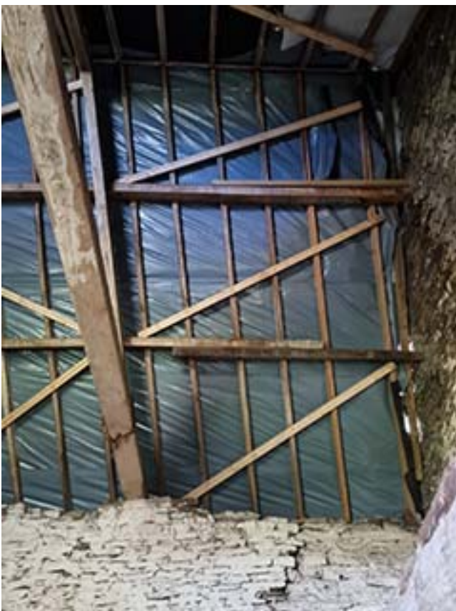
Photo showing misshapen roof structure
