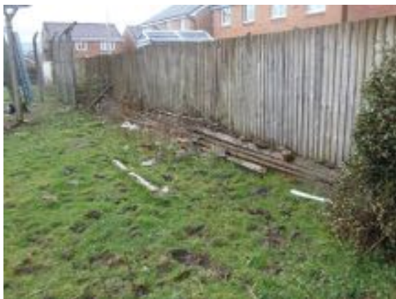
Wooden fencing along western boundary, rubbish
