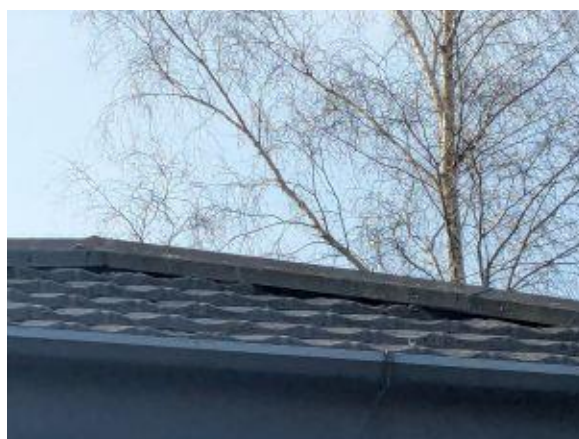
PRFs – gaps present between roofing tiles and ridge.
