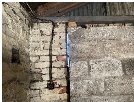
Plate 10: Gap in north-west gable end wall
