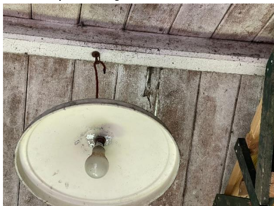
Plate 9: Gaps in ceiling - smaller room
