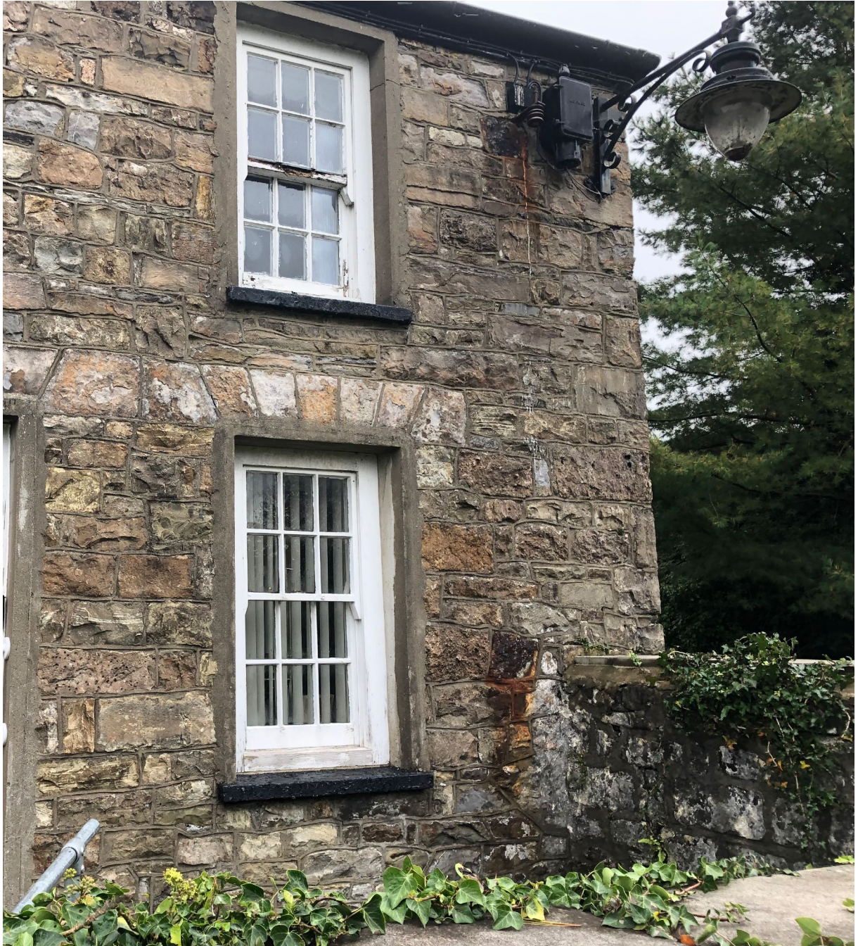
Photo 4 – Windows – First floor window in poor condition
