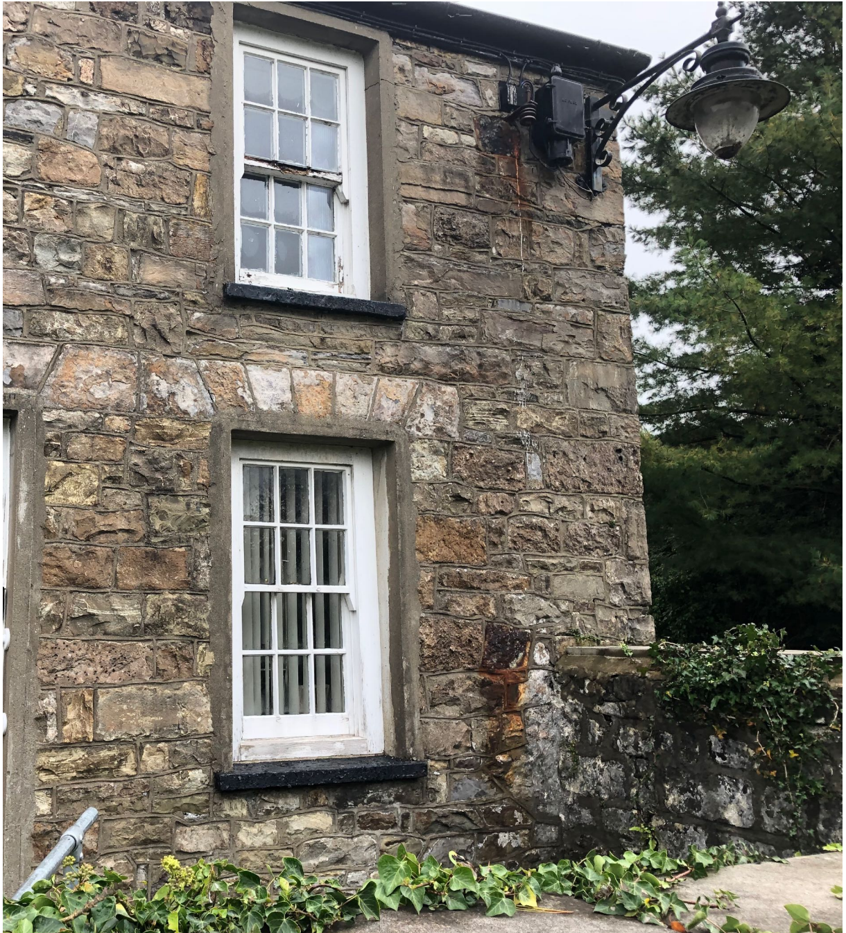
Photo 3 – Windows – First floor window in poor condition
