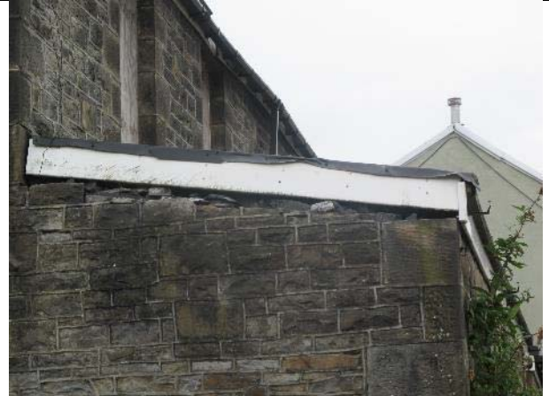
Gaps under PVC fittings on northern extension of building 1
