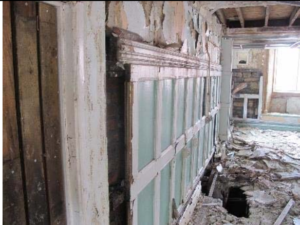
Water damage in building 1 interior
