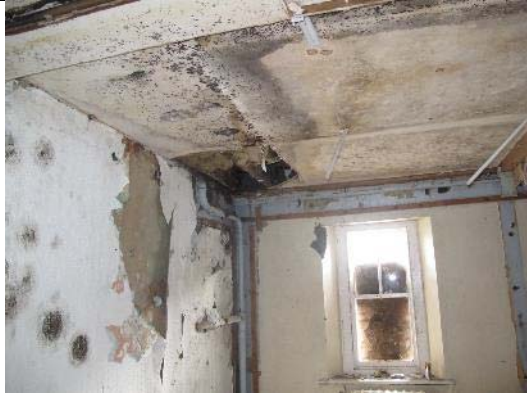
Interior of building 1, water damage
