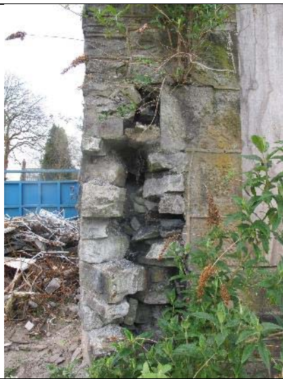
Damage to external stone work on northern extension of building 1
