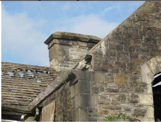
Damage to exterior stone work on western elevation
