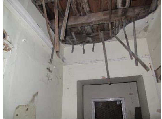
Damage to ceiling, interior of building
