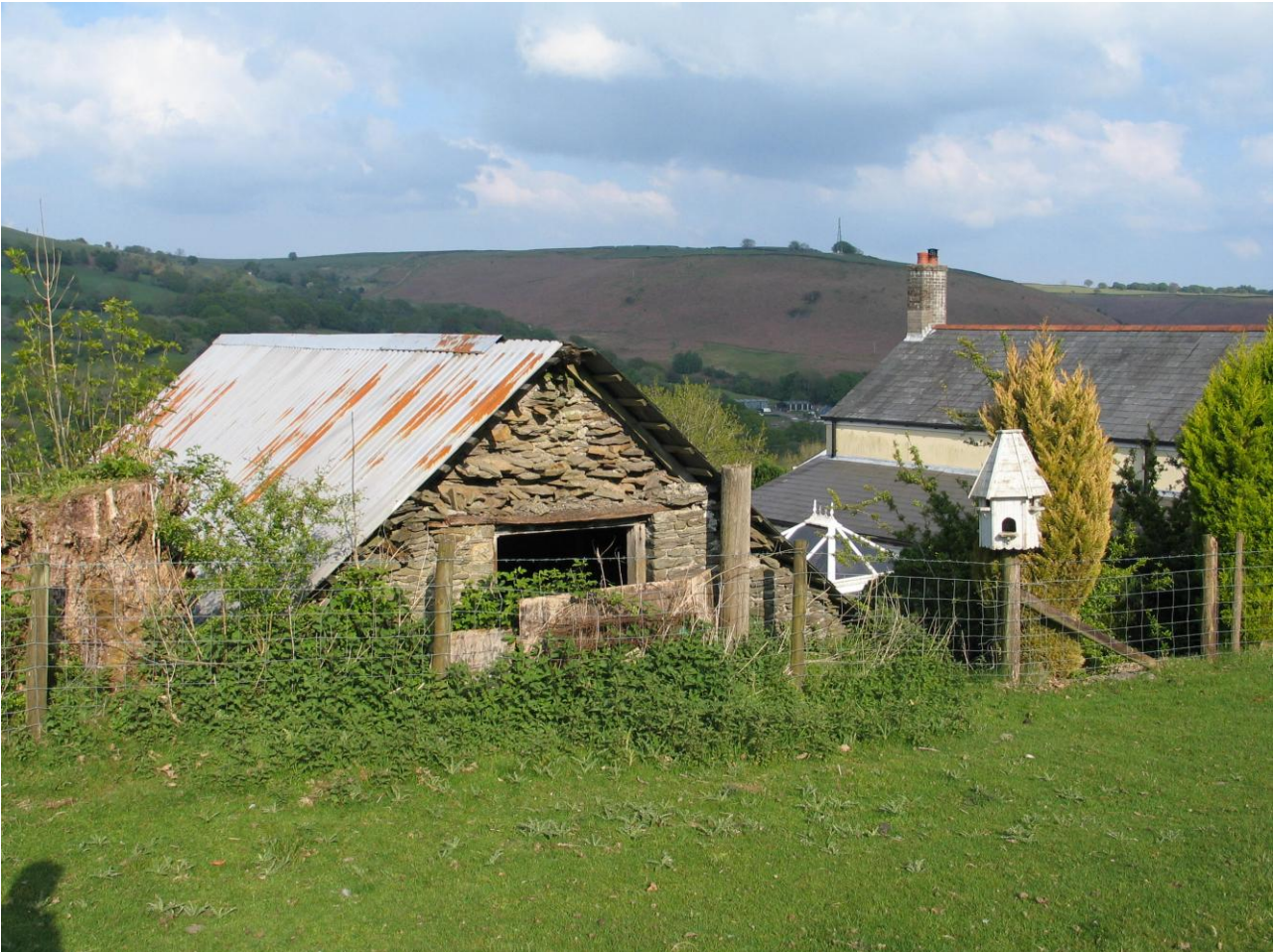
West gable showing missing high level stonework
