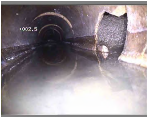
1, 00:00:40, 2.50 m Hole in drain/sewer at joint, from 3 to 4 o'clock
