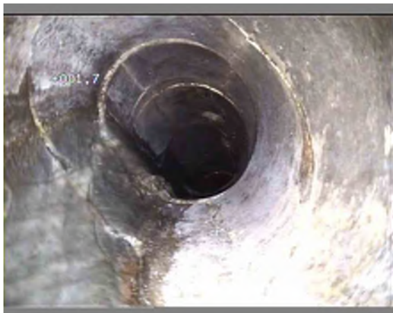
1, 00:01:22, 1.70 m Fracture, circumferential, from 5 to 5 o'clock
