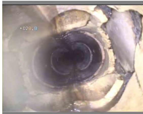
2, 00:05:05, 28.80 m Hole in drain/sewer, from 10 to 2 o'clock
