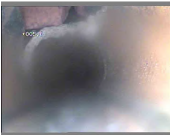
1, 00:01:17, 5.60 m Hole in drain/sewer, from 10 to 2 o'clock
