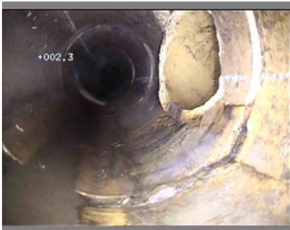
1, 00:00:33, 2.30 m Connection intruding, at 2 o'clock, diameter 150mm, intrusion 5%
