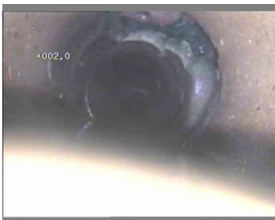
1, 00:00:49, 2.00 m Hole in drain/sewer at joint, from 10 to 3 o'clock
