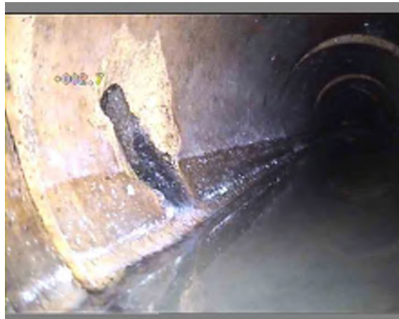
2, 00:00:54, 2.70 m Hole in drain/sewer at joint, from 8 to 9 o'clock
