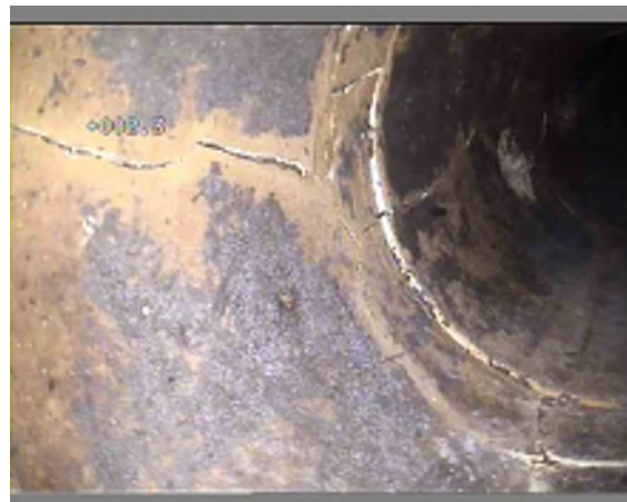
2, 00:01:59, 2.30 m Fracture, longitudinal at joint, at 11 o'clock
