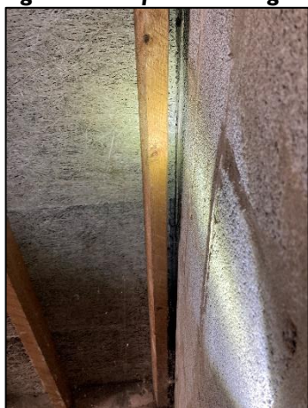
Figure 5 – Gap to rear of garage units
