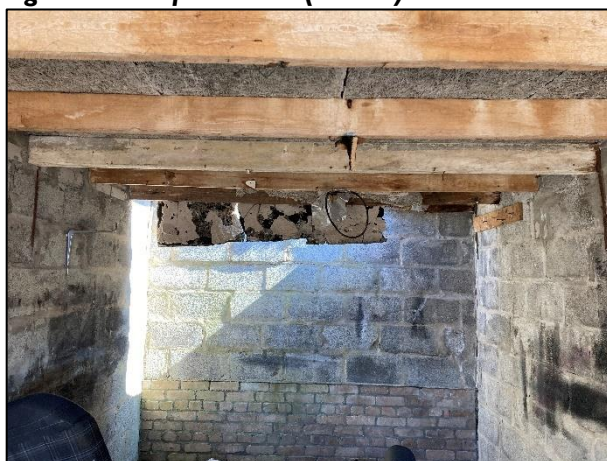
Figure 6 – Collapsed roof (unit 20)
