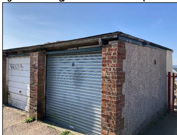
Figure 2 – Missing/rotten wooden frame (units 8 & 9)
