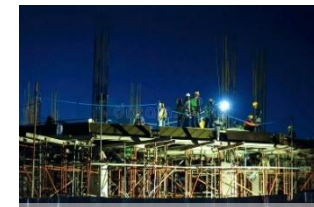
Fig.3.12 – Local task lighting
