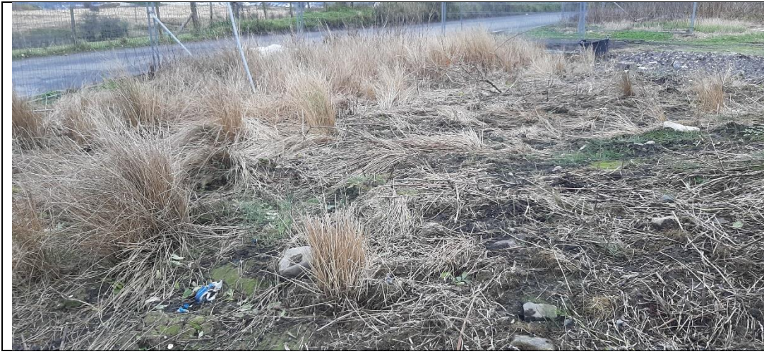
Photo 8. Rushes of a former sewage soakaway
