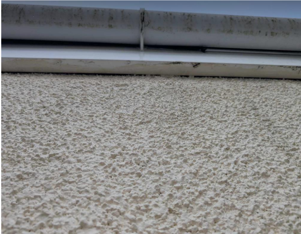
Plate 7- photograph of gap beneath fascia board of extension
