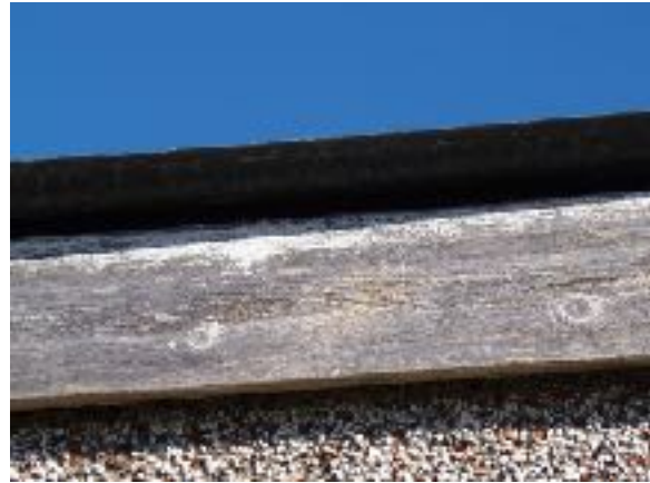
B2 – gap under fascia
