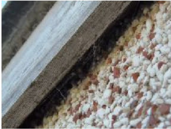
B2 – gap under fascia with cobwebbing
