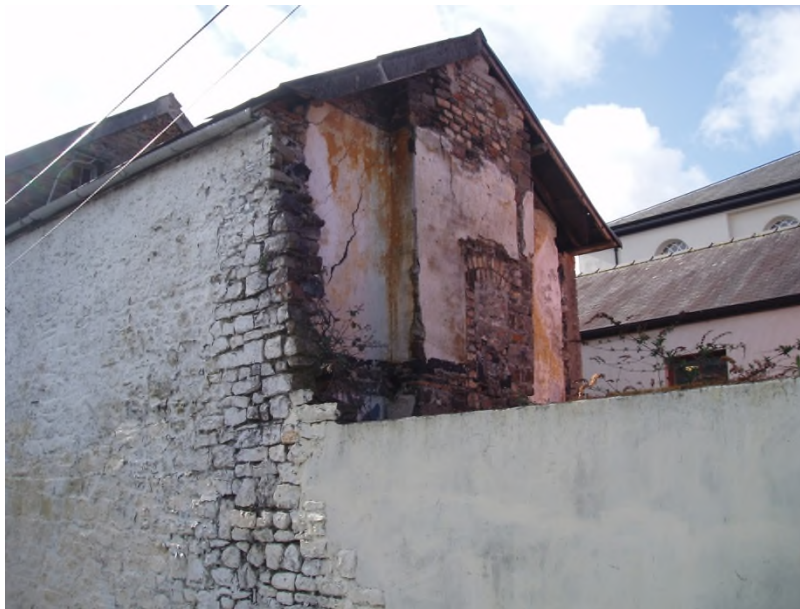
Part of the extensive damage to the one end (nearest Nant Morlais) of the property
