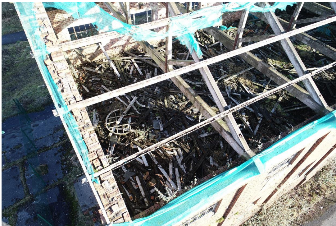
Photograph 13 ~ Roof debris on first floor level to west end
