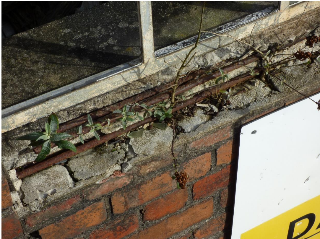
Photograph 28 ~ Corrosion of metal reinforcement bars causing concrete lintel to disintegrate
