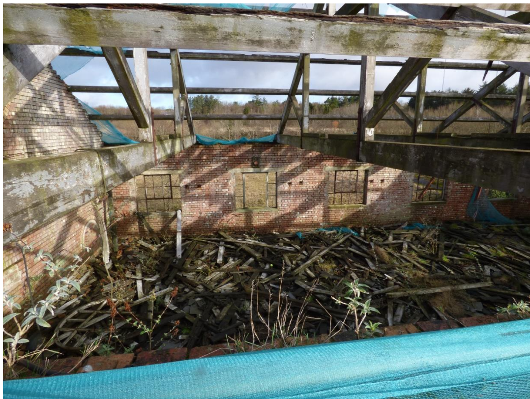
Photograph 20 ~ Roof debris on first floor to west end
