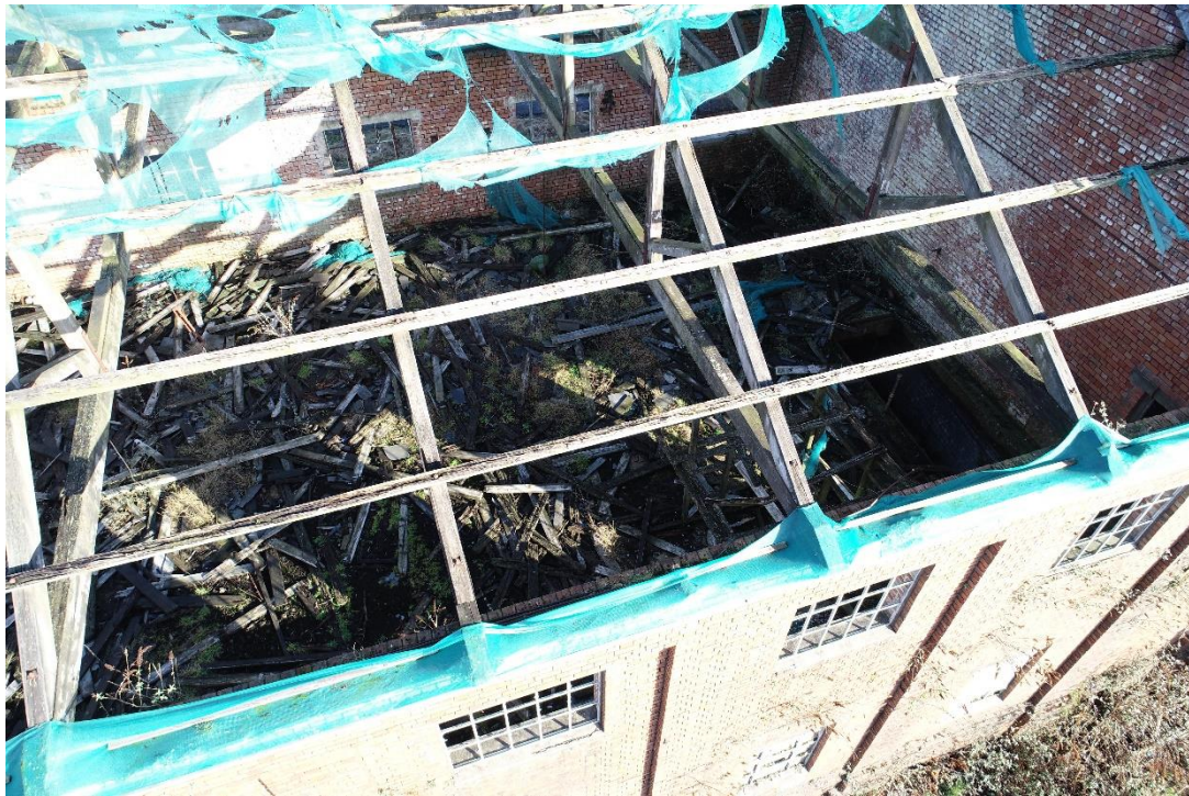
Photograph 14 ~ Roof debris on first floor structure to west end
