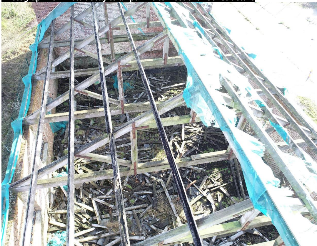
Photograph 15 ~ Note decay to all purlins to west end roof structure
