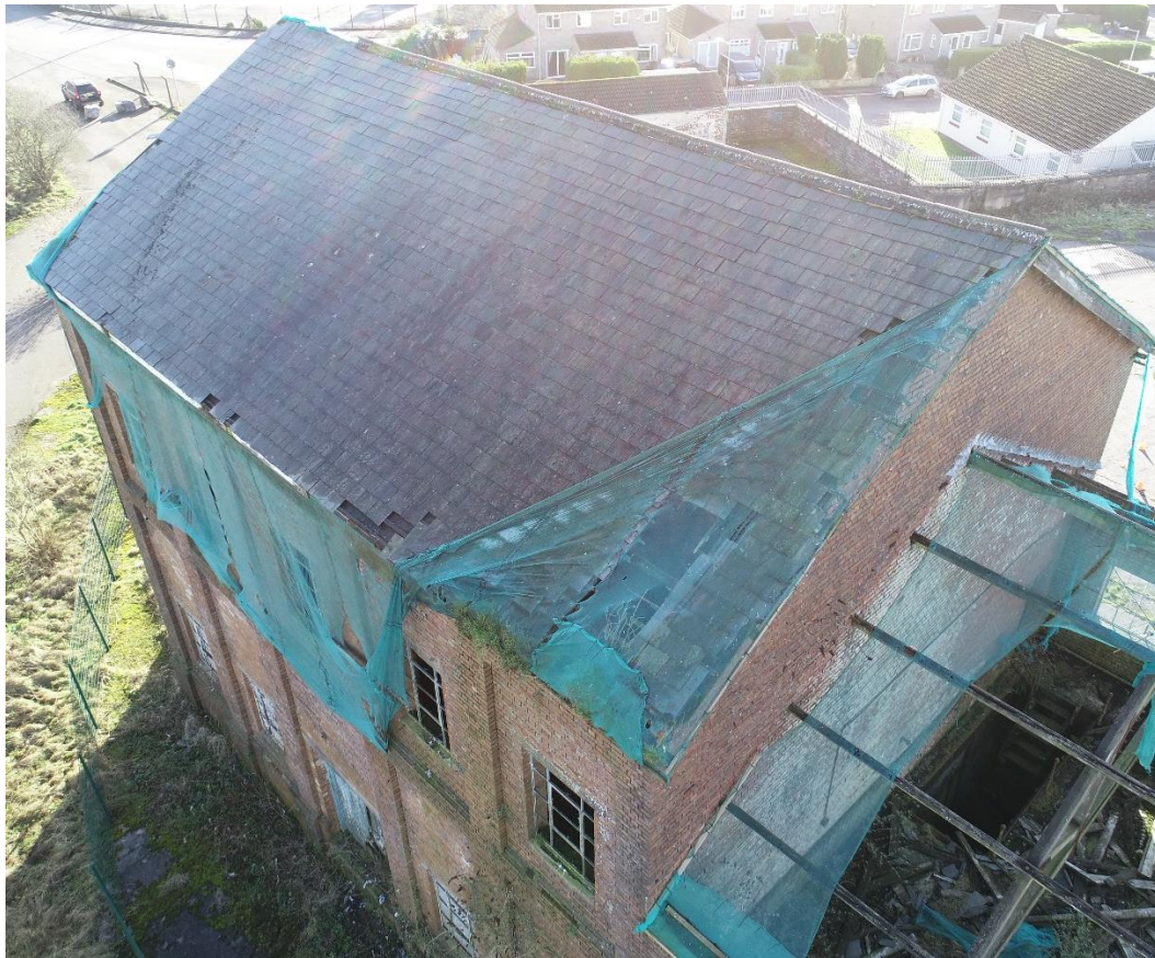
Photograph 16 ~ Roof holed to rear elevation under netting
