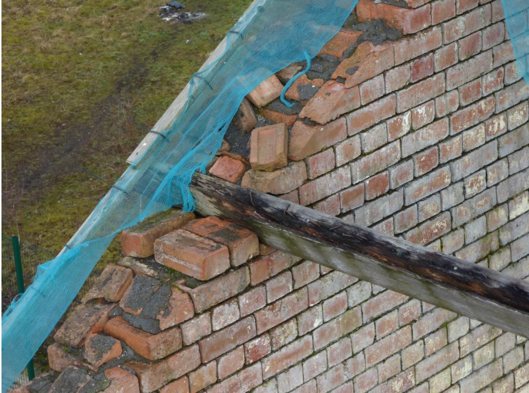
Photograph 22 ~ Loose bricks to west end gable wall purlin loosely supported
