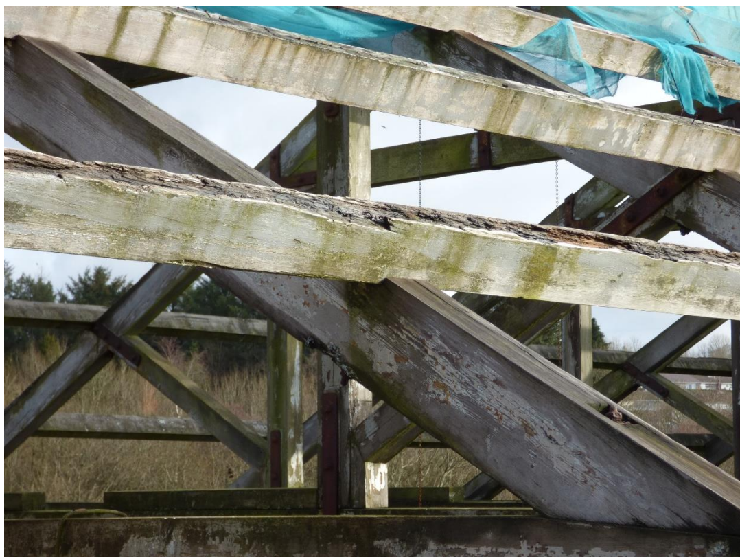
Photograph 18 ~ Decay to purlins where bolted to truss
