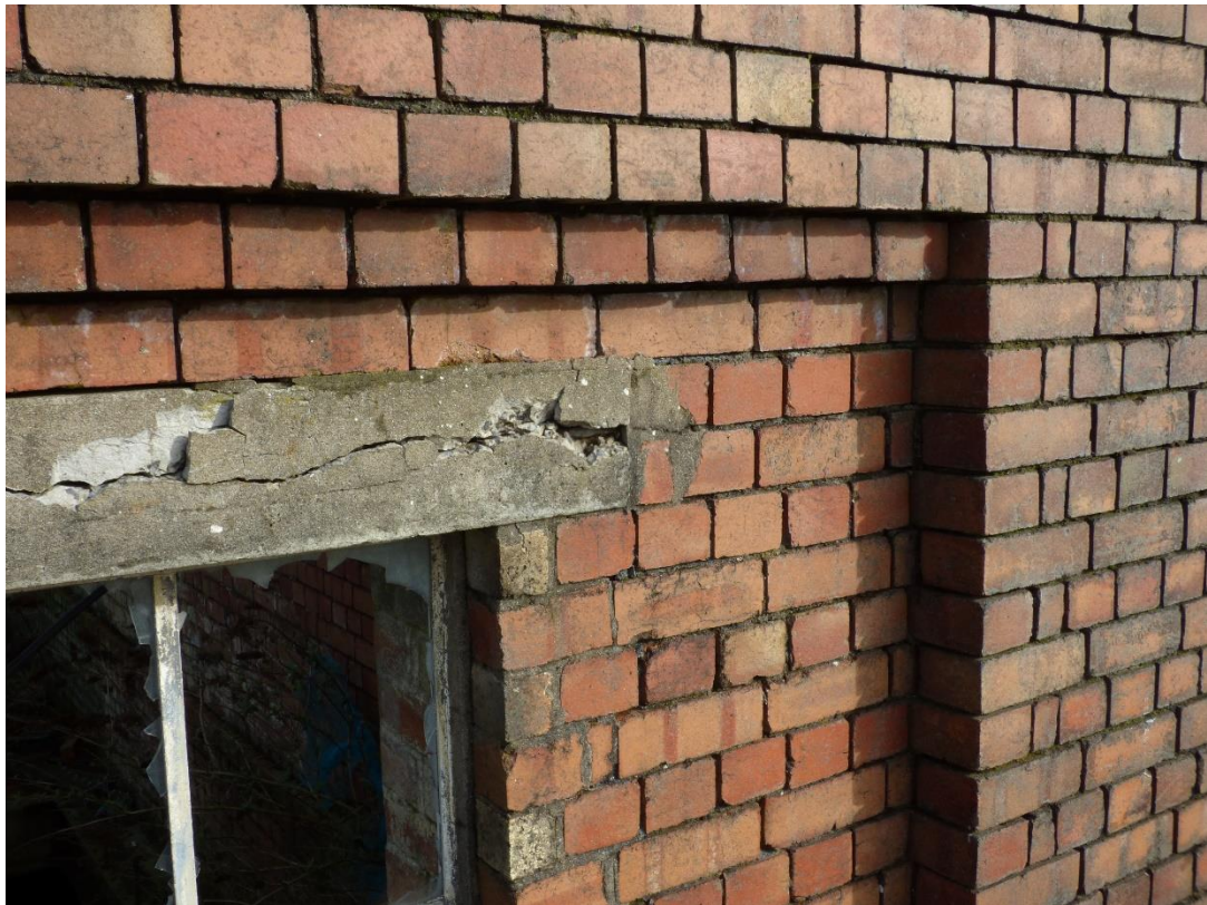
Photograph 27 ~ Typical deterioration to precast concrete lintel
