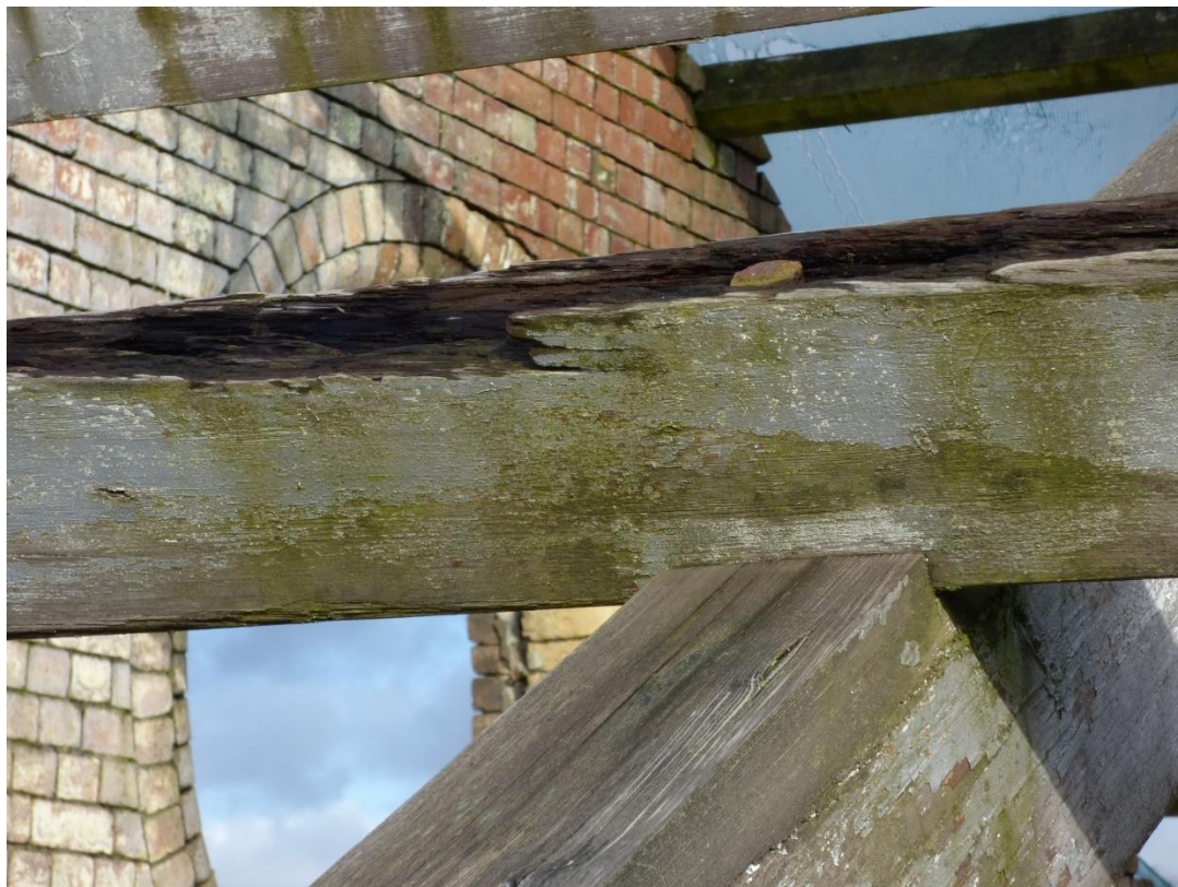
Photograph 19 ~ Decay to purlin where bolted to truss
