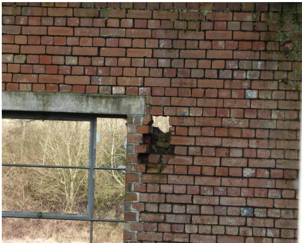
Photograph 26 ~ Internal view of hole in wall as above
