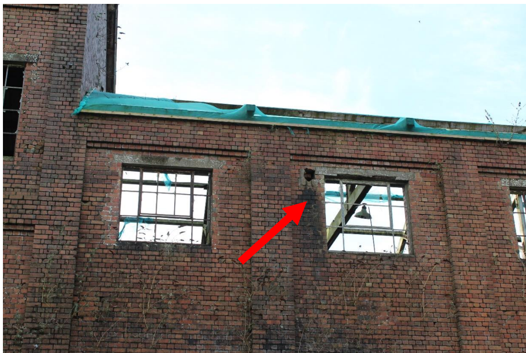
Photograph 25 ~ Hole in wall and deterioration to rear elevation lintel
