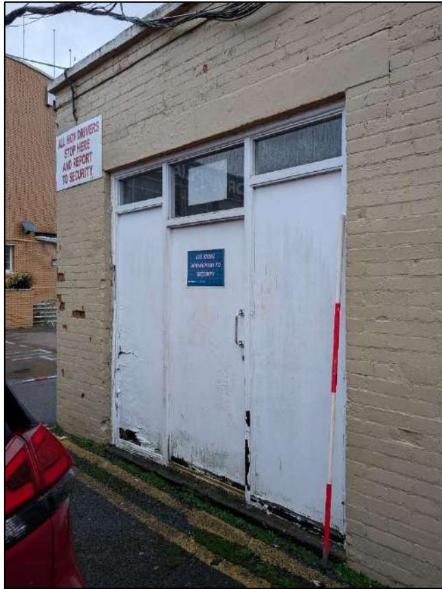
Plate 27. Left rear door, view to the north.
