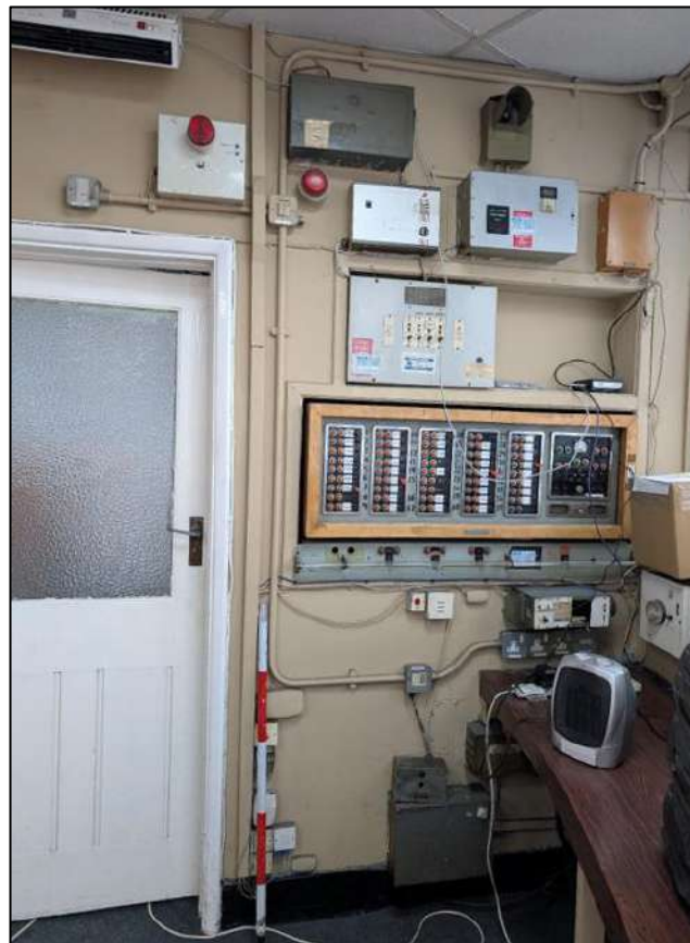
Plate 34. Doorway to electrical room showing control panels, view to the west.
