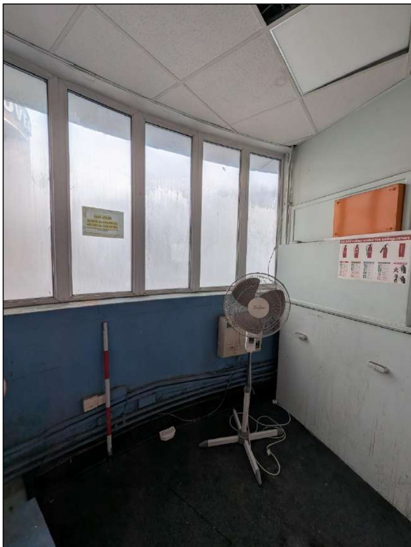
Plate 45. Electrical room, view to the north.
