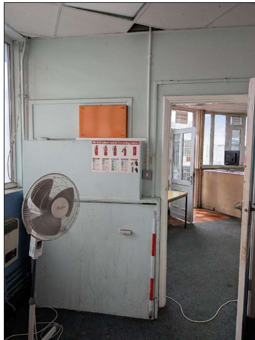
Plate 46. Electrical room, view to the east
