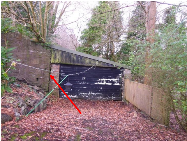
Figure 11: Garage (missing mortar in brickwork)
