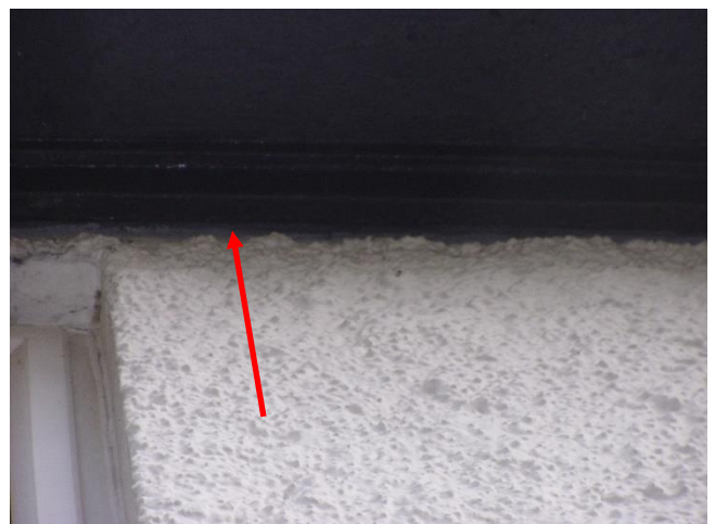
Figure 10: Gap between soffit box and wall
