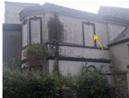
Plate 2 – Southern elevation showing blocked up windows. Arrow showing gaps between the blockwork and window opening.
