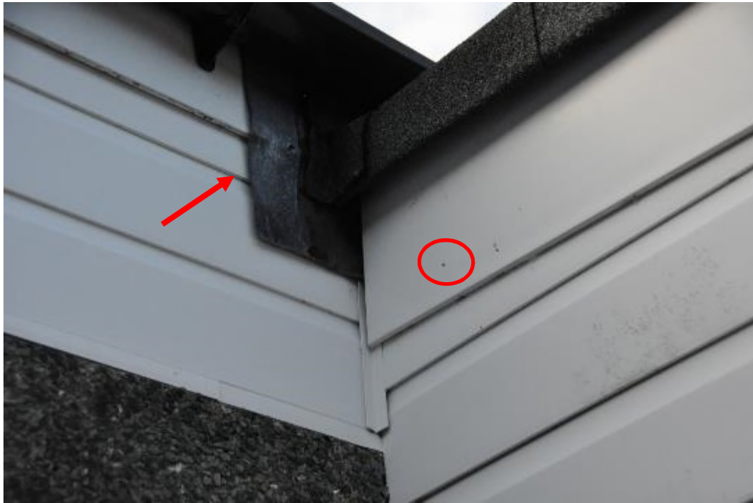
Plate 9 bat dropping recorded on fascia and roost recorded behind lead flashing
