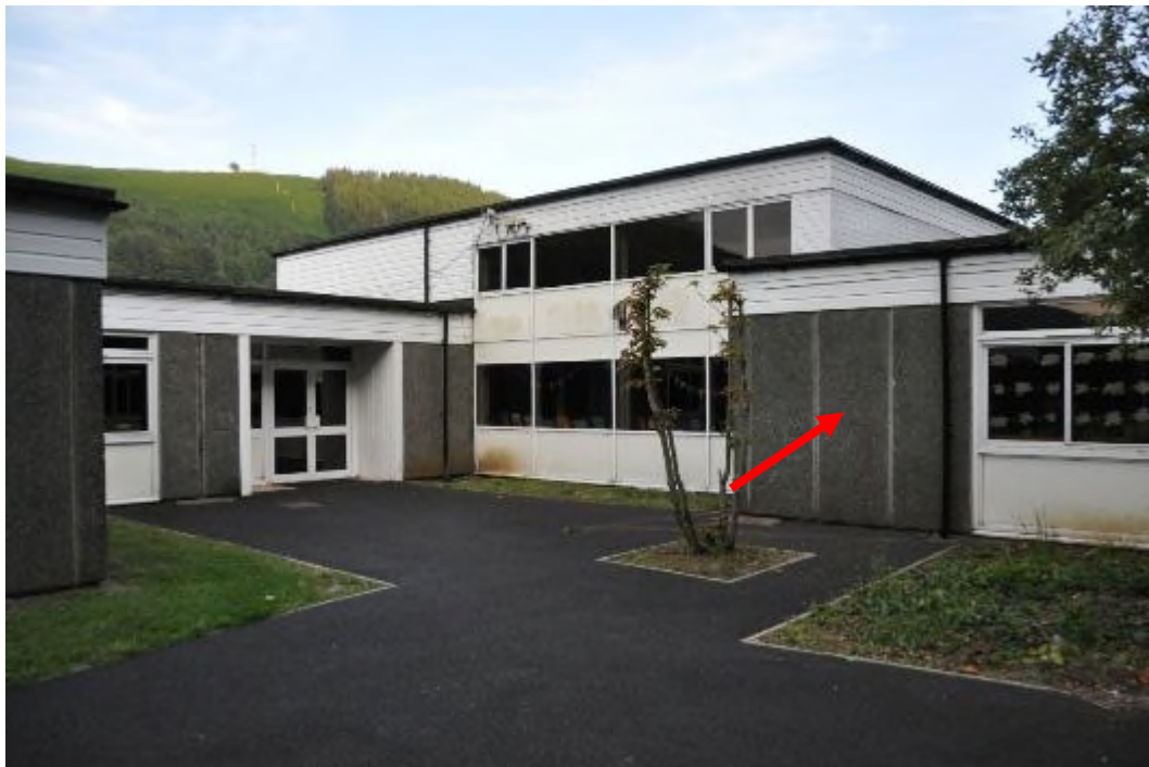
Plate 6 some concrete panels had gaps but no evidence of use by bats
