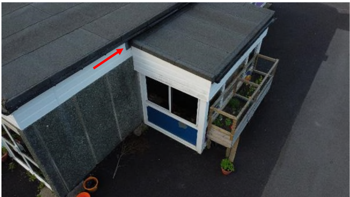
Plate 4 showing area of small soprano pipistrelle day roost behind lead flashing
