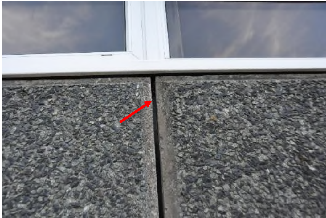
Plate 7 showing gaps between concrete panels no evidence of use by bats
