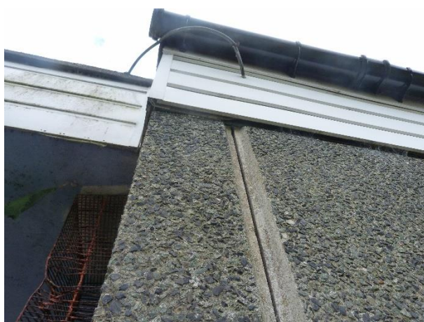
Photo 9: Gaps under uPVC fascias on eastern aspect
