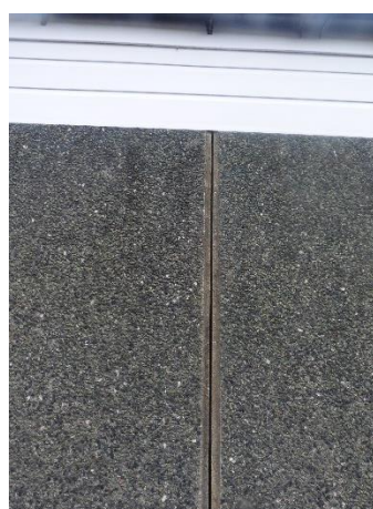
Photo 10: Gap in concrete cladding on eastern aspect
