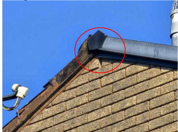
Photo 8: Gap at apex on southern elevation and missing mortar between bricks
