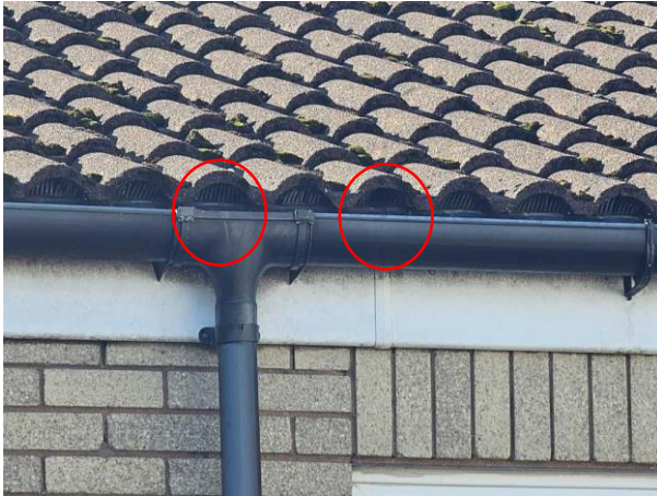
Photo 7: Interlocking tiles with missing wildlife spikes
