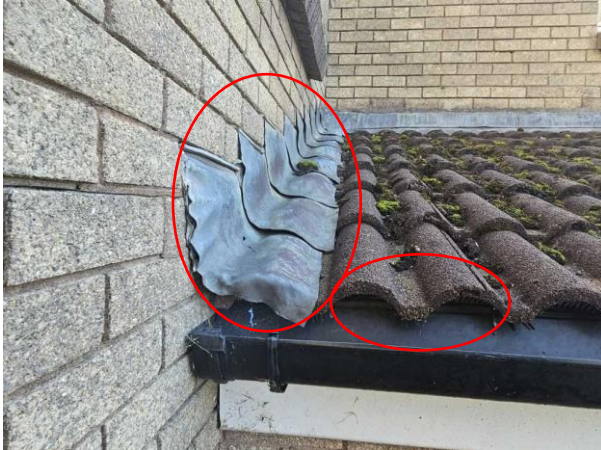
Photo 9: Lifted led flashing and missing wildlife spikes
