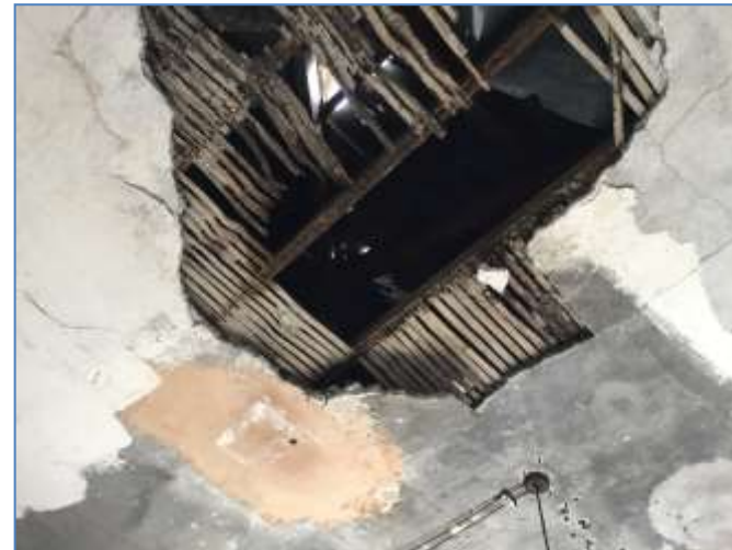
Photograph 24. Building E. Damage to the ceiling showing the unlined roof above and access through the roof.
