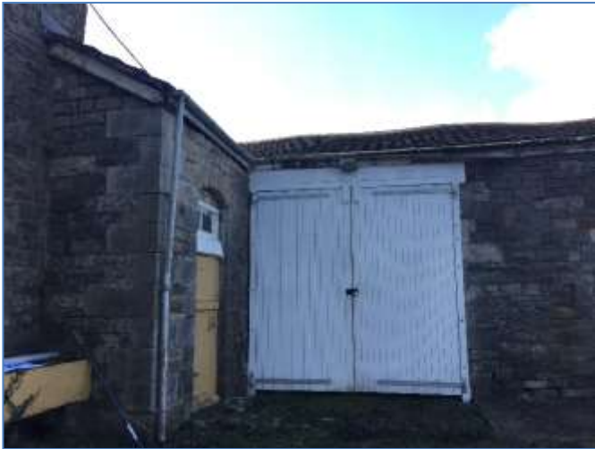
Photograph 33. Building G. Gaps beneath fascia boards at the western corner.
