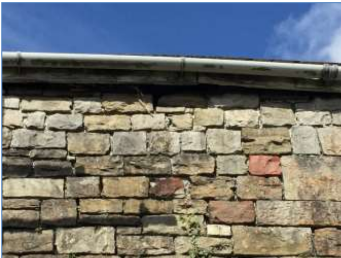
Photograph 35. Building G. Significant gaps beneath fascias on the eastern elevation.
