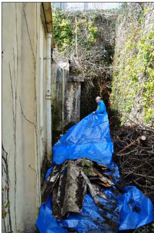
Plate 10. Asbestos storage to side of the east side walls
