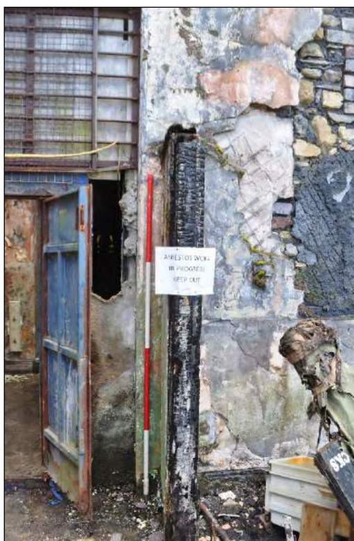
Plate 15. Close up of doorway (west interior) into Church hall with burnt original doorframe
