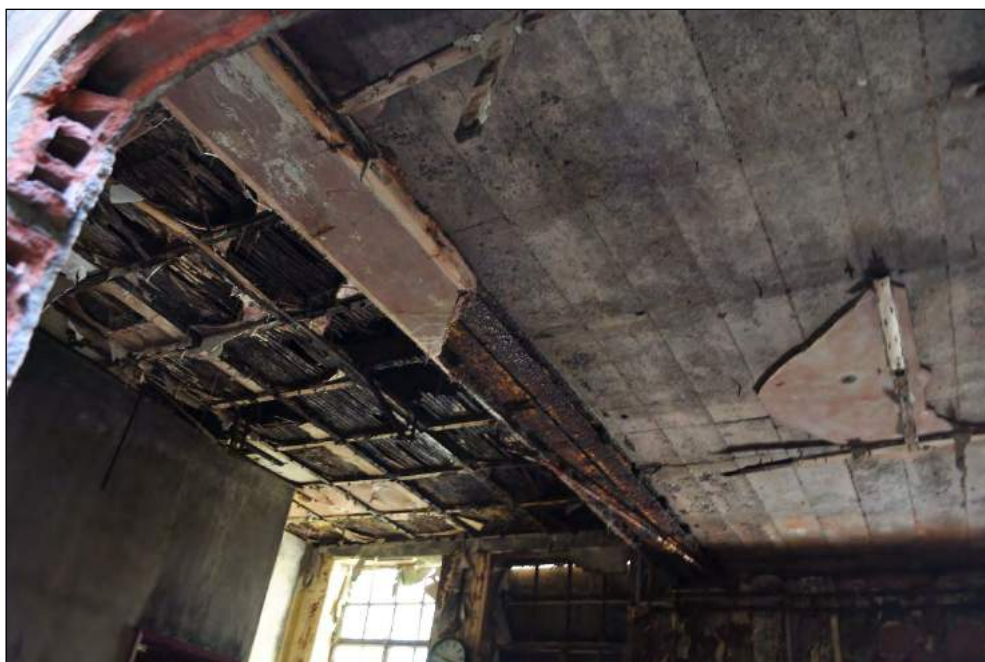
Plate 32. Concrete ceiling with burnt out fittings the first room accessed within the Labour Exchange fronting the road looking south (the clock had survived the fire)
