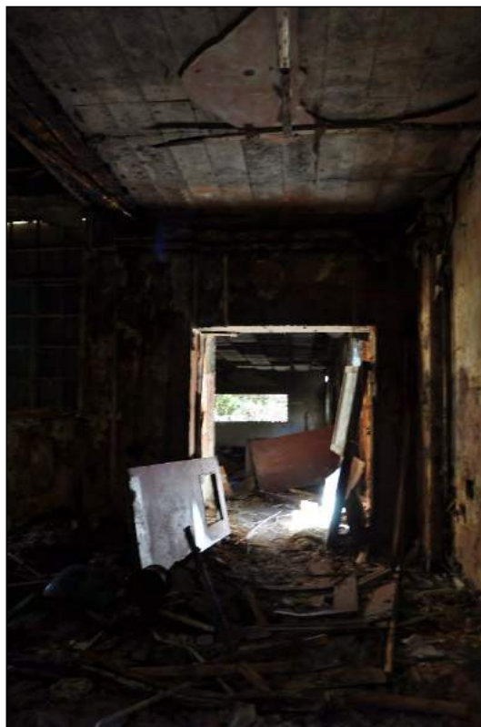
Plate 33. Show the level of debris within rooms looking west towards exterior wall of building
