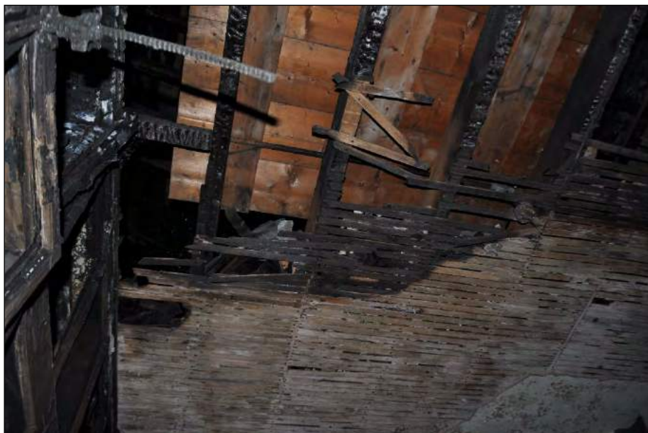
Plate 35. Fire damage to ceiling in Labour Exchange building
