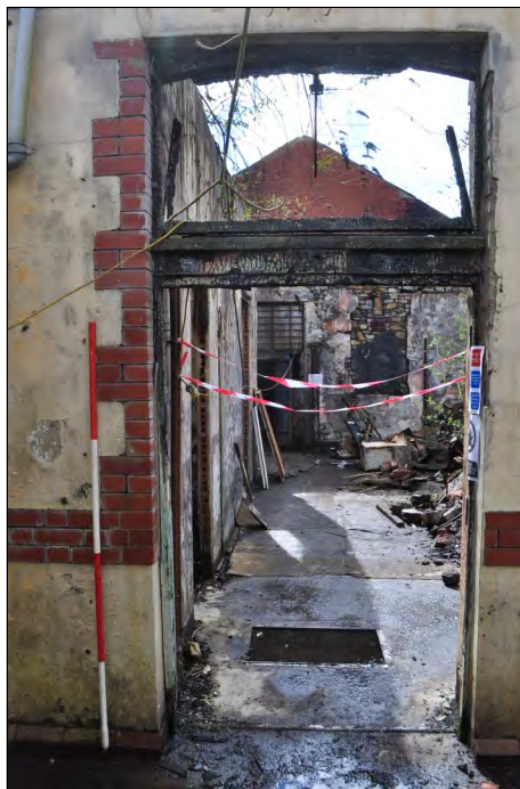
Plate 12. Close up of burnt out entrance doorway (east side) into Church hall
