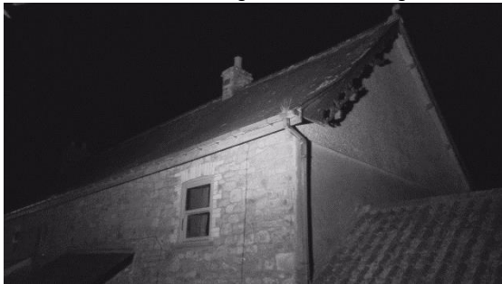
Plate 17: House, infra-red image of north-western gable
