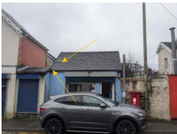
Eastern elevation – PRF – raided leadwork, slipped slates, raised slates.
