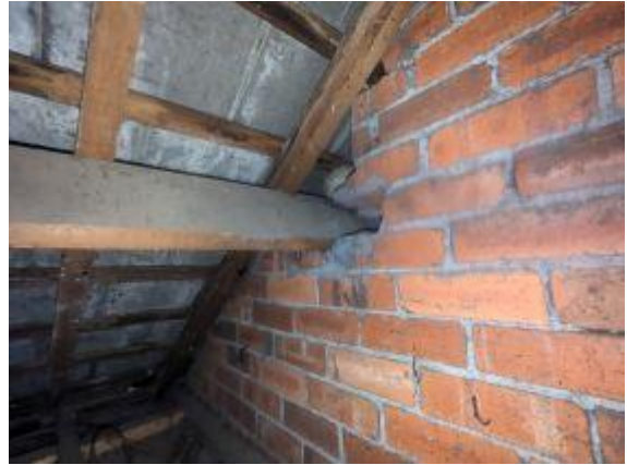
PRFs – Cavity above bitumen membrane.
