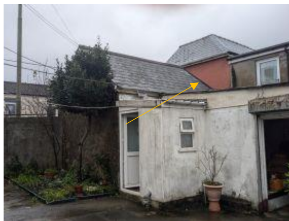
Western elevation – PRF – gap along edge of roof.
