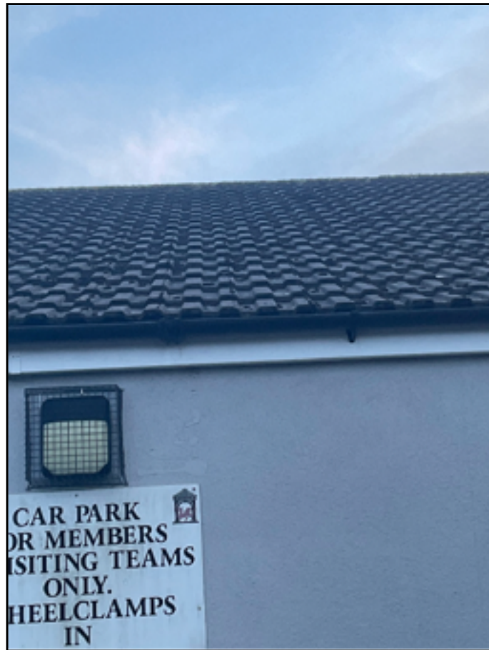
Areas of Missing Mortar Between Tiles
