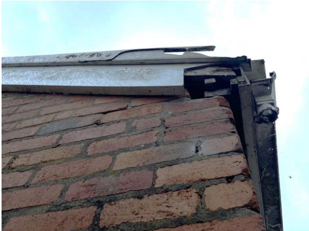
Photo 18: Broken uPVC Plastic Trim on the Eastern Elevation
