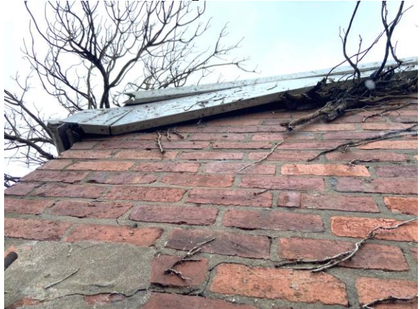
Photo 19: Lifted Upvc Bargeboard on the Eastern Elevation of the Building
