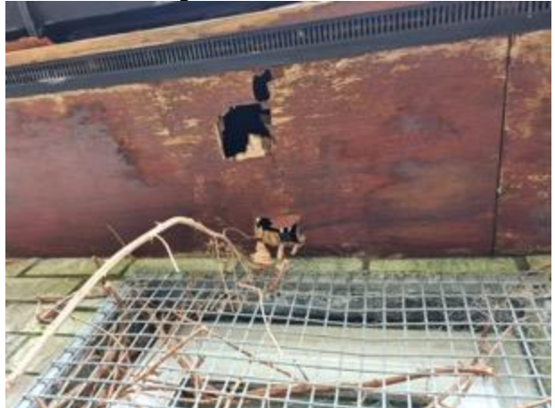
Photo 12: Damaged Timber Soffit Box
