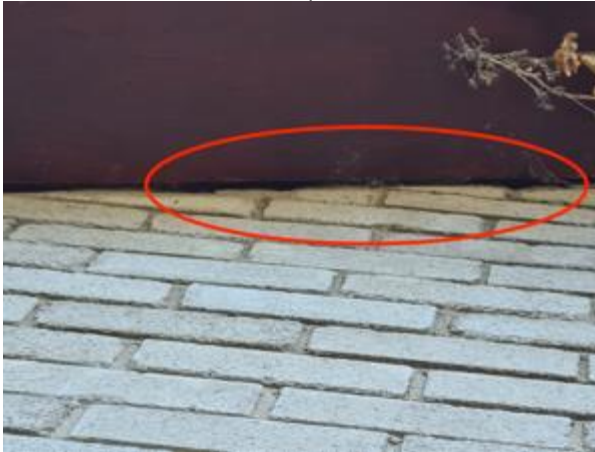
Photo 9: Lifted Timber Soffit Box from Brick Wall on the Southern Elevation, Circled
