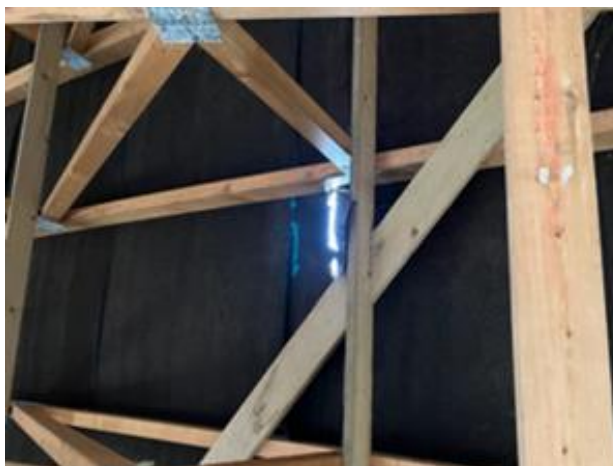
Photo 19: Tear in Bitumen Felt Roof Lining
