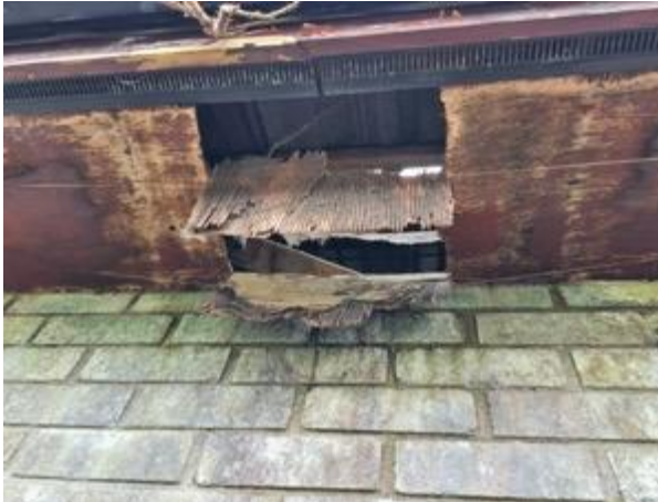
Photo 11: Broken Timber Soffit Box
