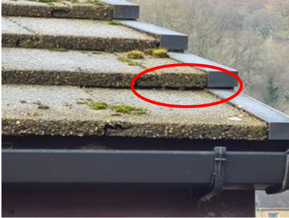
Photo 7: Eastern Elevation Lifted Roof Tile, Circled
