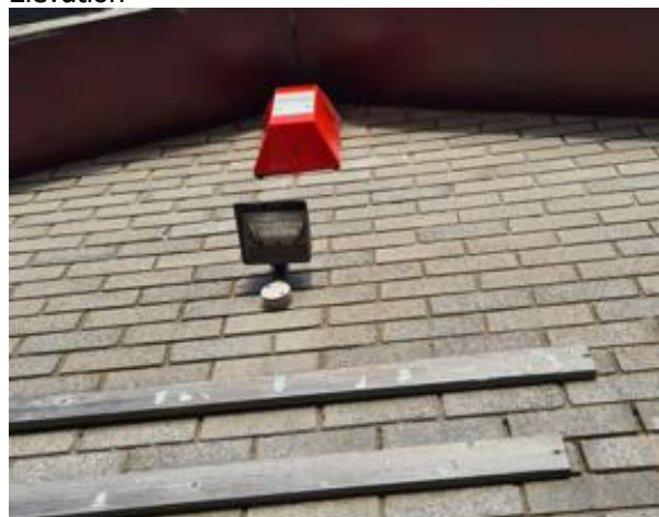
Photo 20: Smashed Security Light, on Southern Elevation
