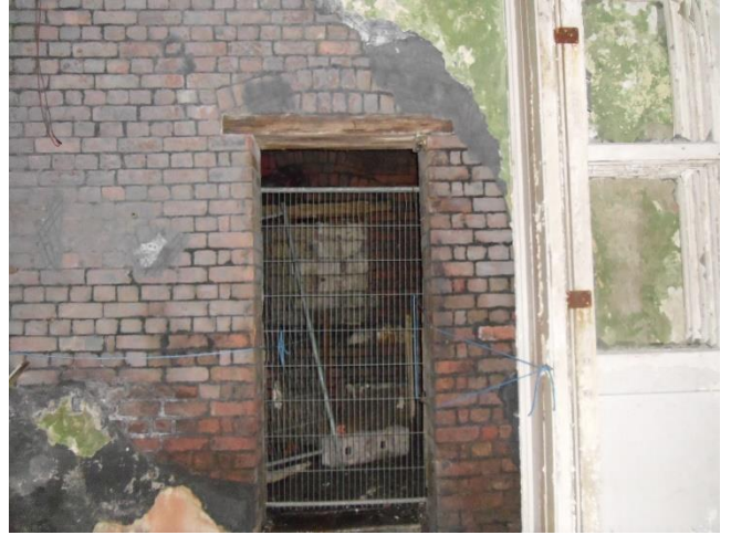
Figure 15 - Fenced off door at rear of building
