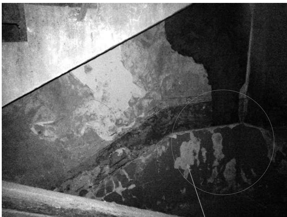
Fig 8 Showing the scheme running up the wall of the staircase. Note the damaged surface of the plaster & also later interventions.
