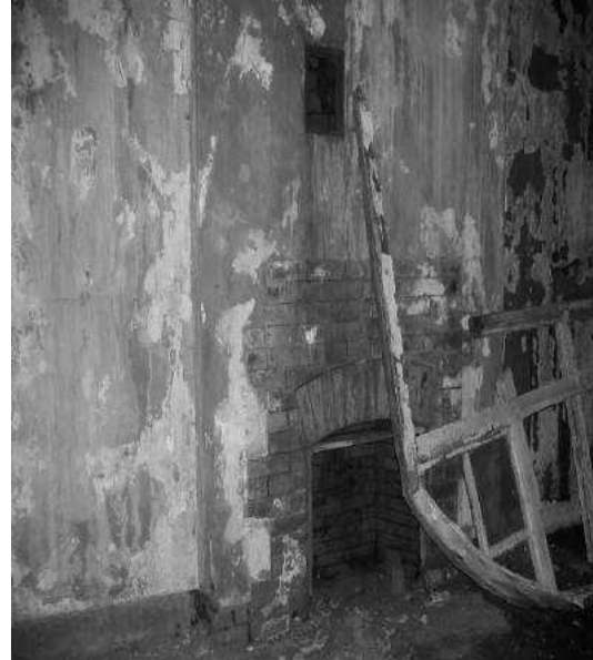
Fig 54 surviving timber window frame
