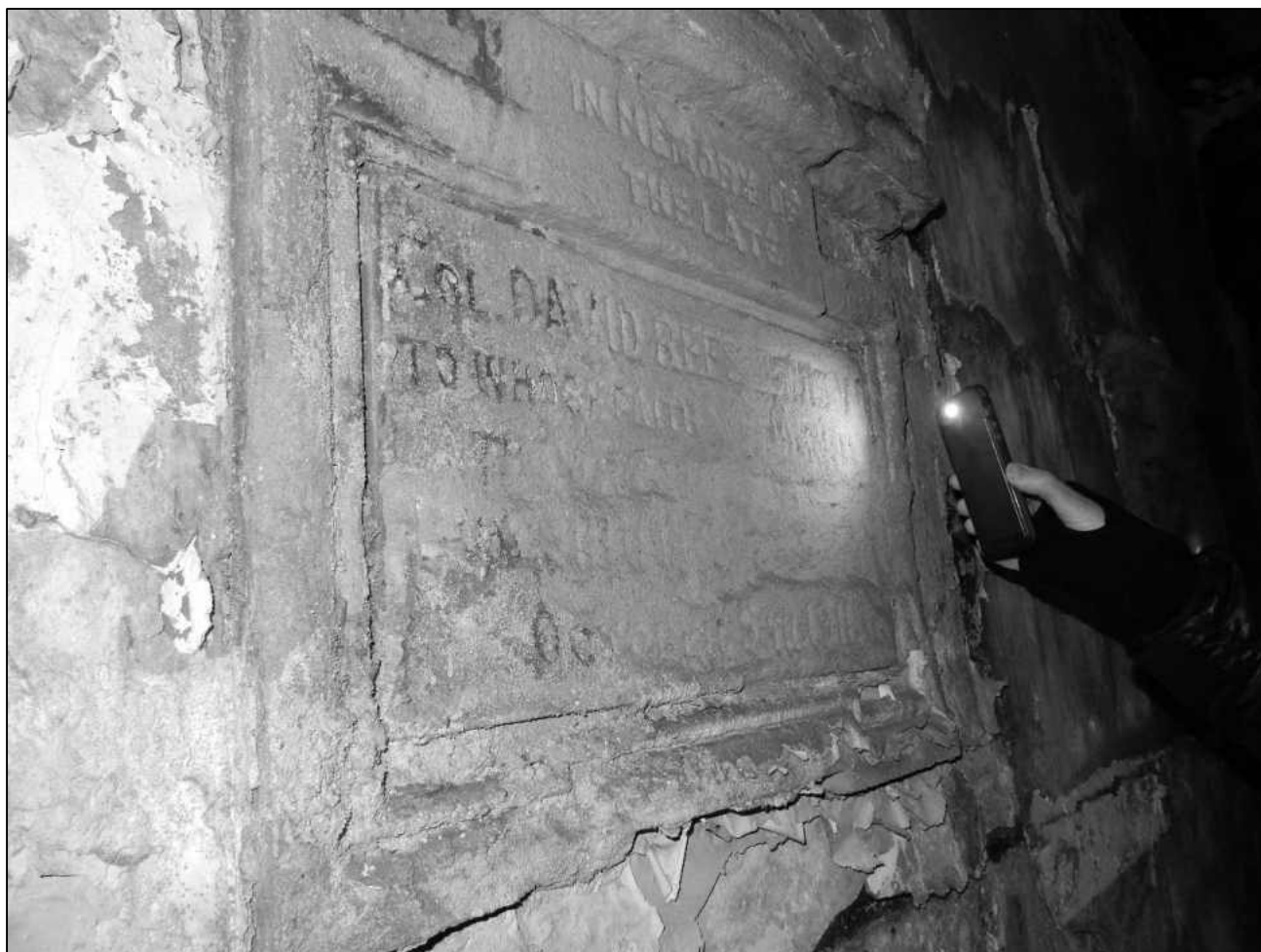
Fig 4 Plaque 2 – evidence of damp and deterioration of the soft limestone.
