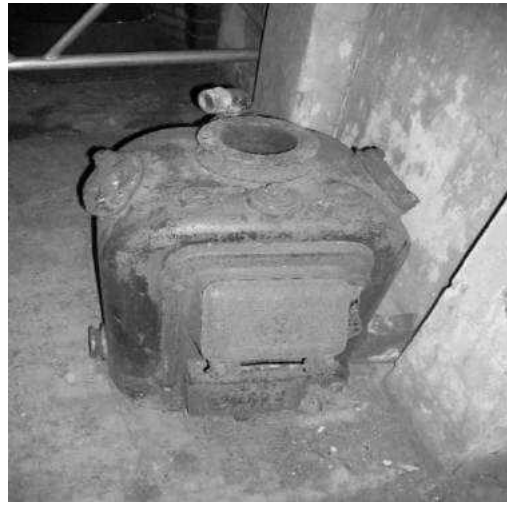
Fig 44 hot water heating system
