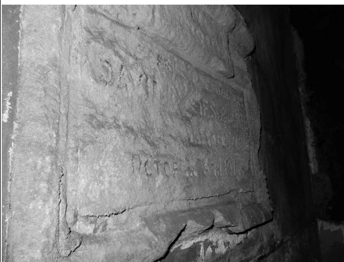
Fig 5 Showing loss of surface and inscription as well as damp coming through the stone and plaster.
