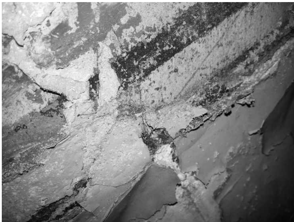
Fig 9 Subsequent paint layers shown peeling back in the damp atmosphere & the (original) black overlaying the brown polychrome layer.
