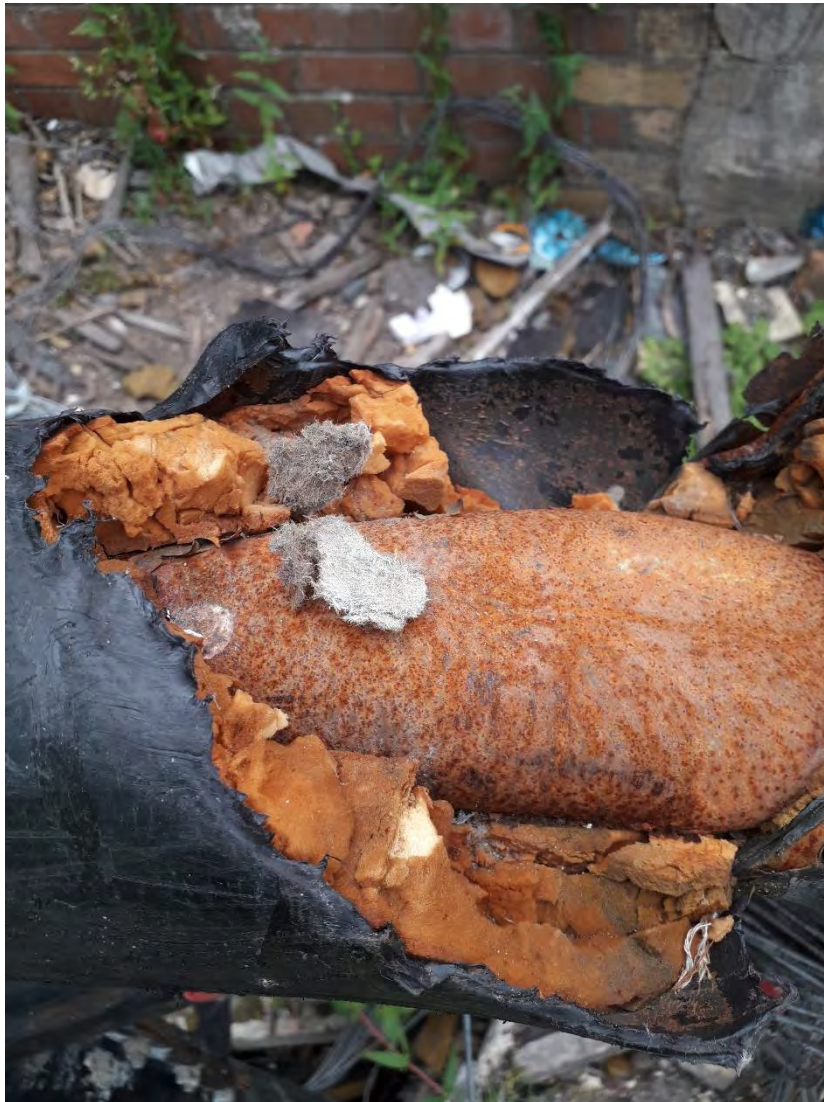
Pipe showing lagging
