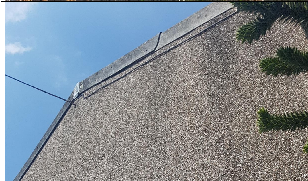
Photo 4. Side gable end (east) with small gaps at the barge board
