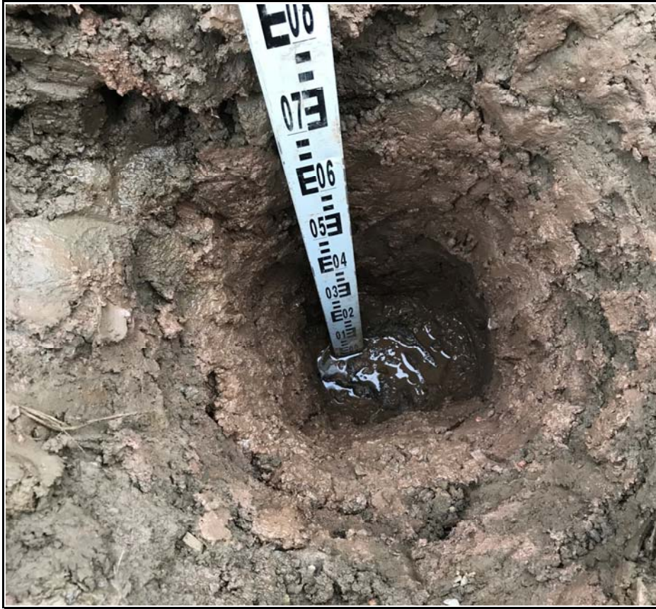
Plot 113 Showing Membrane Placement (Water Ingress)
