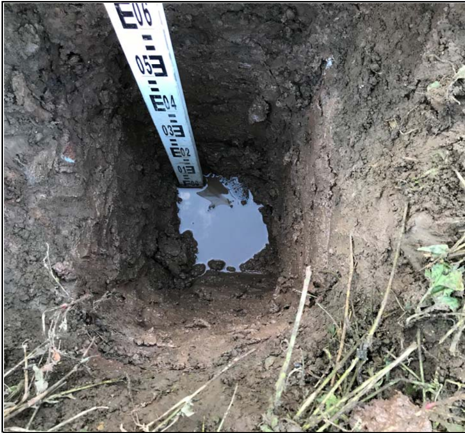
Plot 104 Showing Membrane Placement (Water Ingress)
